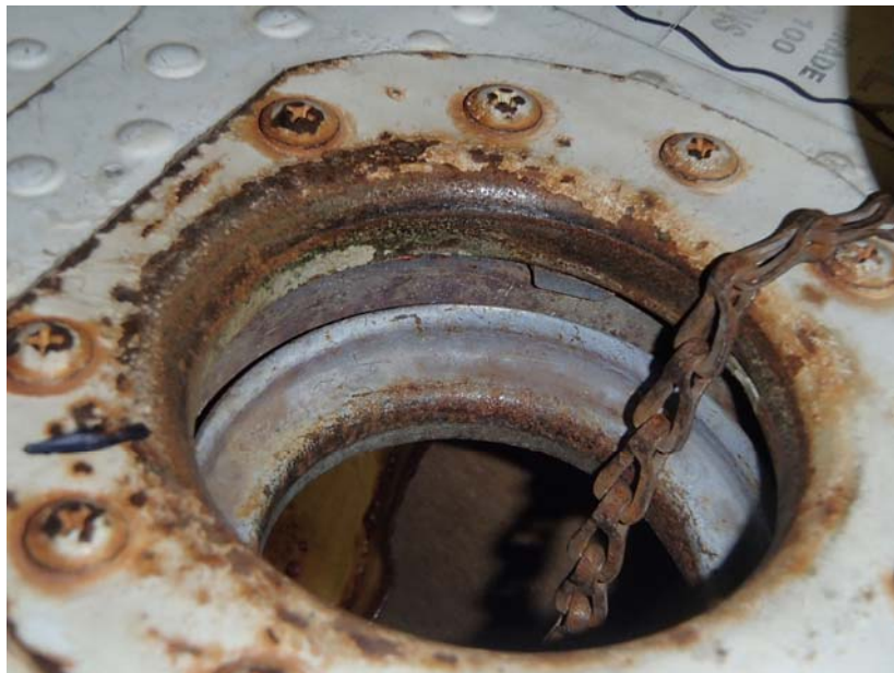
Figure 10 Right fuel tank filler neck showing corrosion and drain channel
