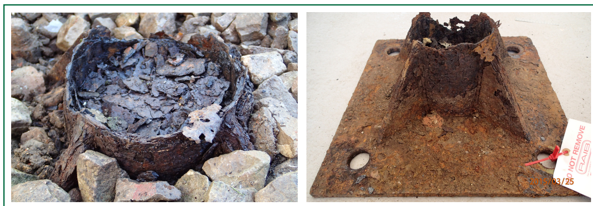
Figure 8: Corrosion at the baseplate (a) in situ after the accident (left image; note level of ballast) and (b) after removal from site
