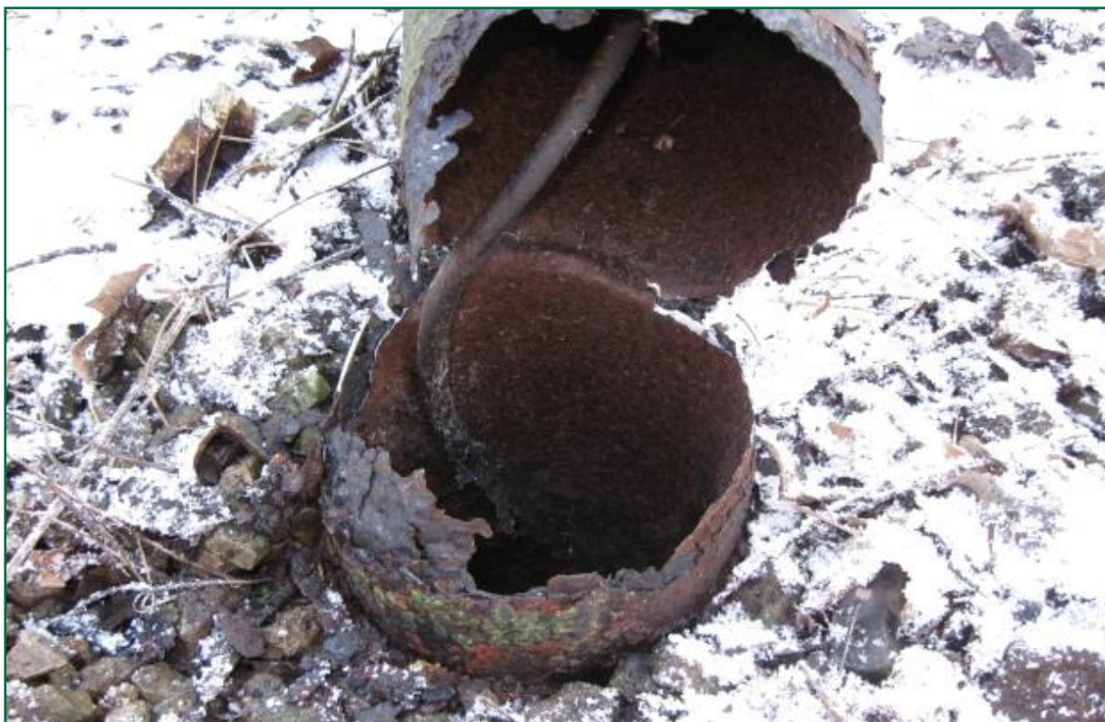
Figure 14: Photograph of the failed signal post at Wymondham (courtesy of Network Rail)
