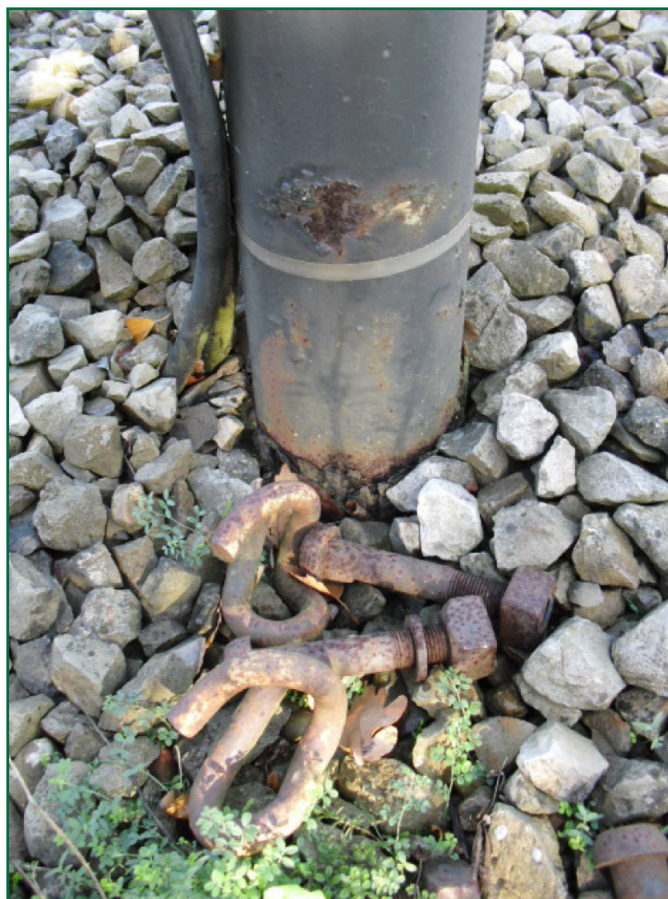
Figure 13: Photograph from Arup's RORI examinations report showing the base of signal TR824
