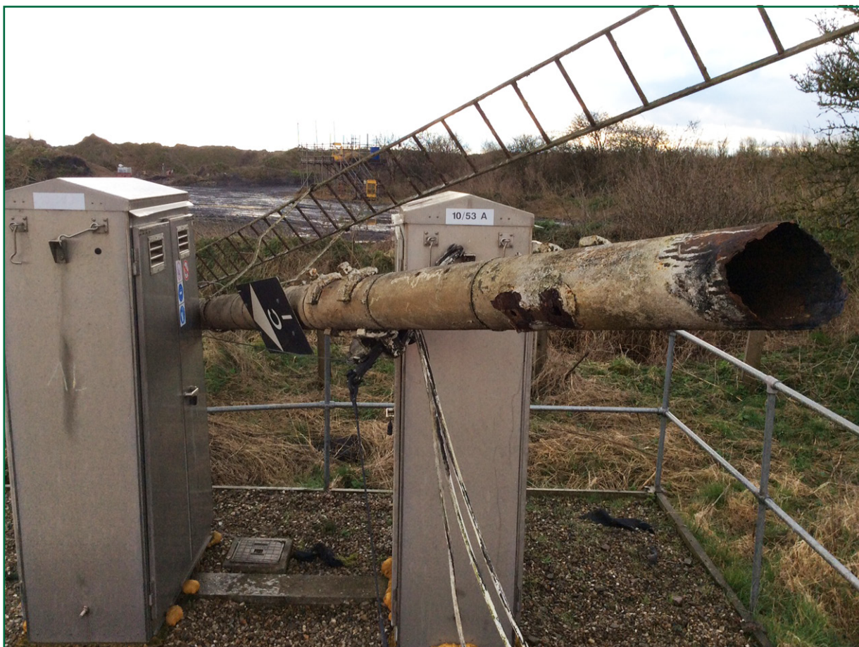
Figure 15: Photograph of the failed signal post at Cantley (courtesy of Network Rail)
