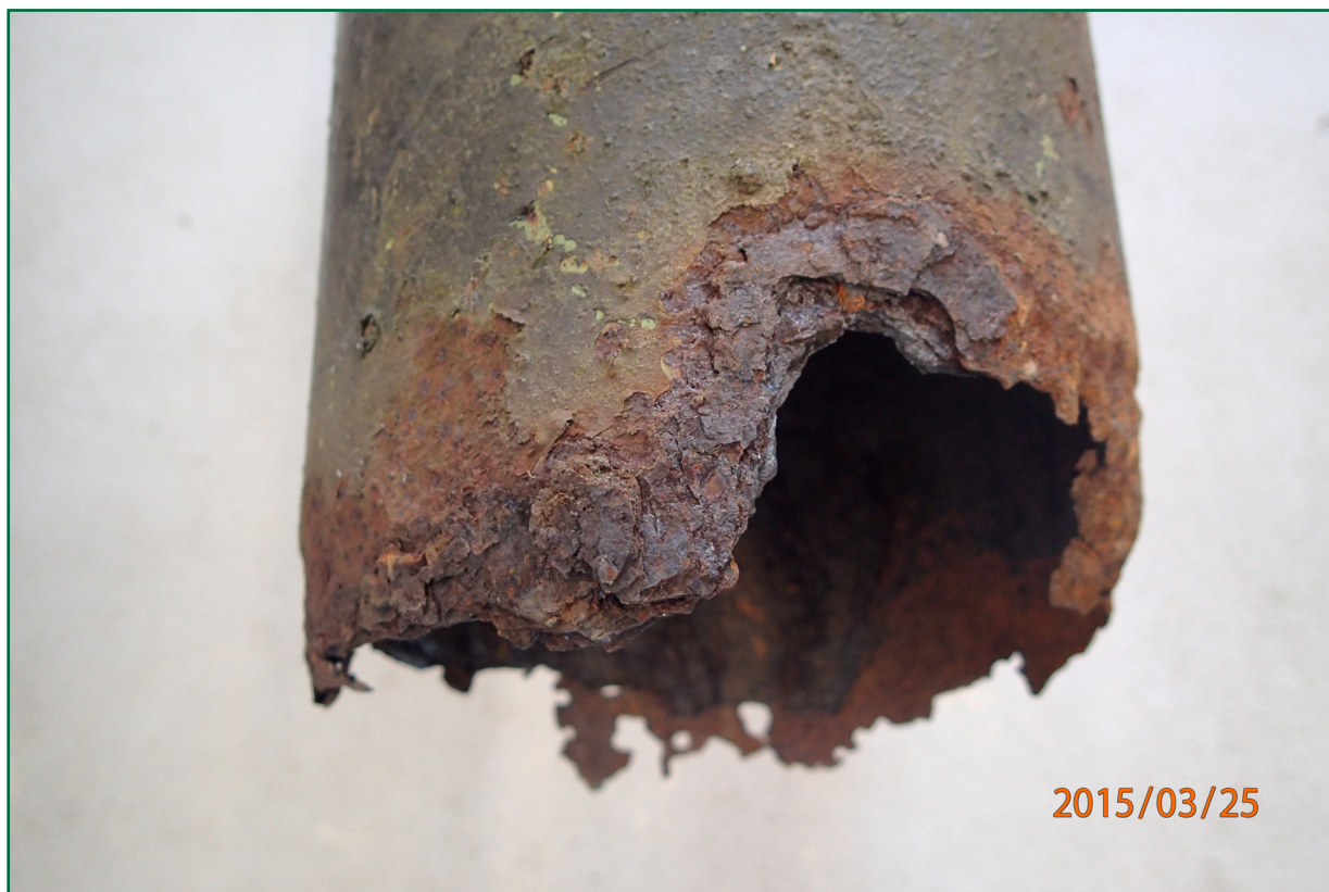
Figure 7: Corrosion at the base of the signal post
