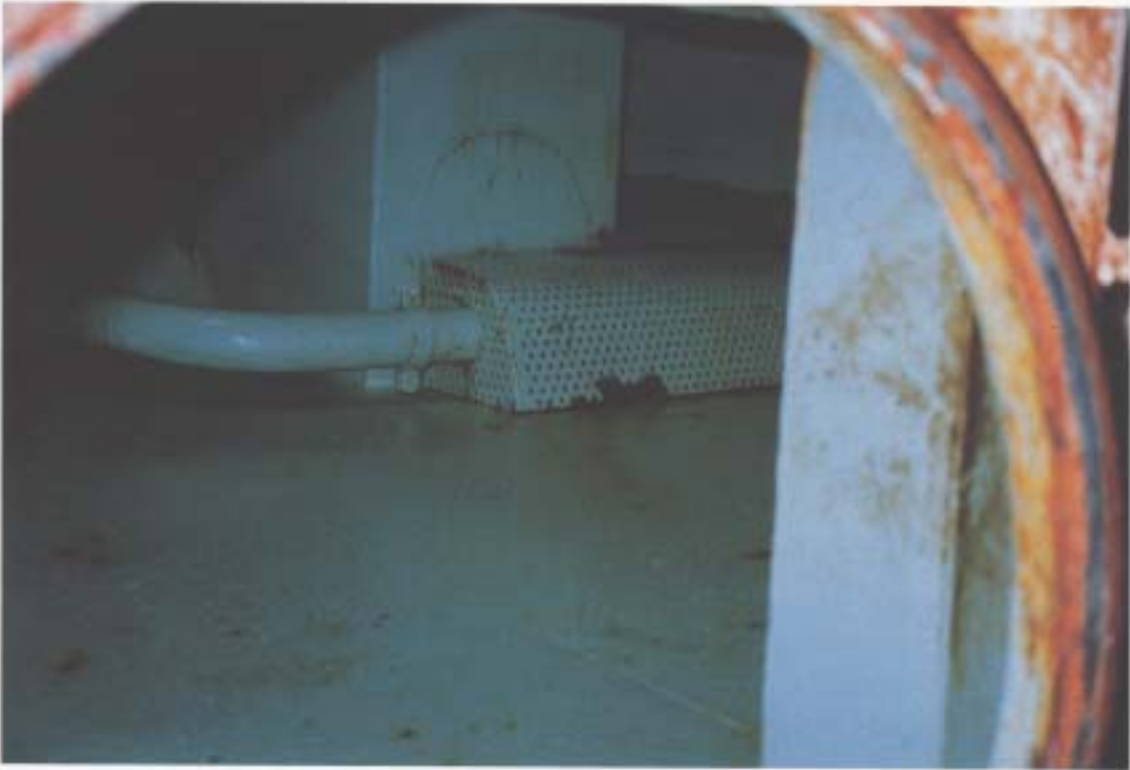
RSW circulating strainer in RSW tank
