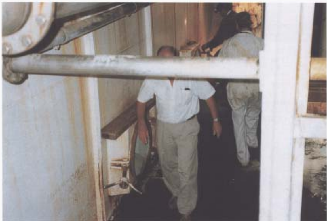
RSW tank side door: partly obscured door is that of No 3 starboard RSW tank
