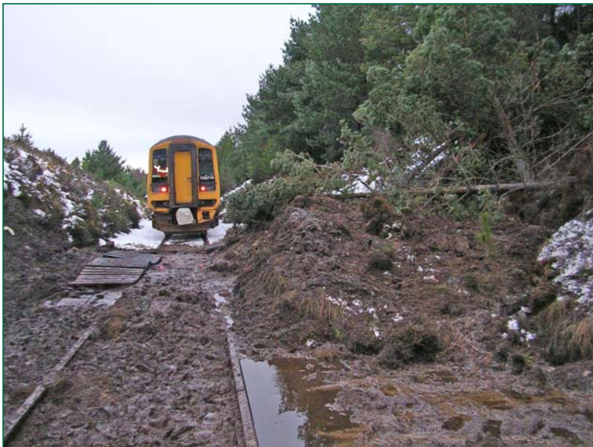
Figure 7: Debris pile from landslip (the train shown is the one sent to site for rescue). (Photograph: Network Rail)
