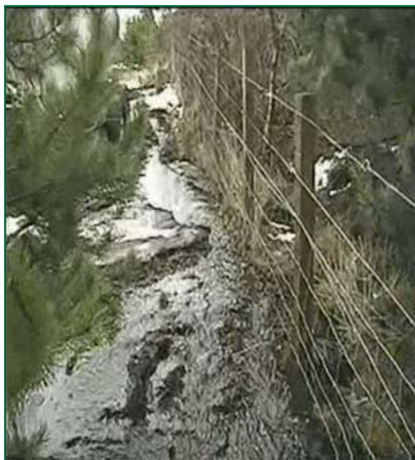
Figure 5: Still image from the site video showing water breach through the boundary fence and into the Network Rail crest drain (Image: Network Rail).
