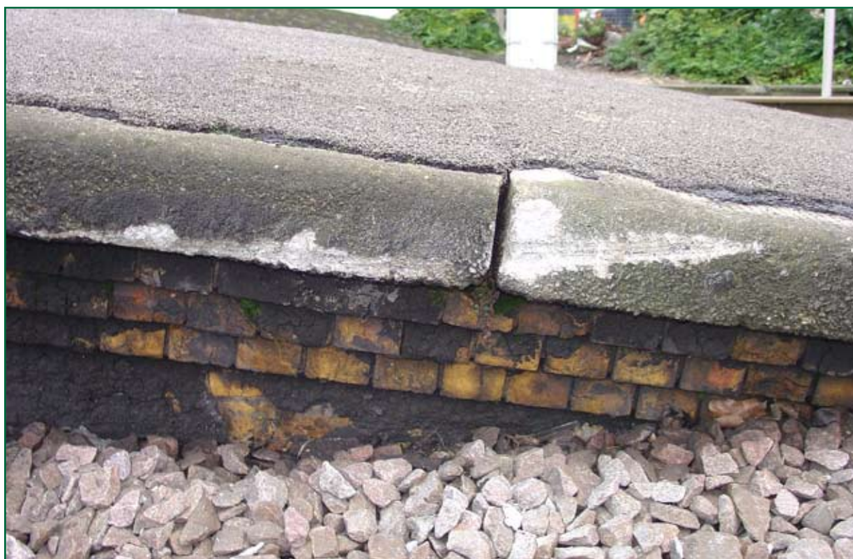
Figure 10 Platform three coping stone misaligned by impact with bogie
