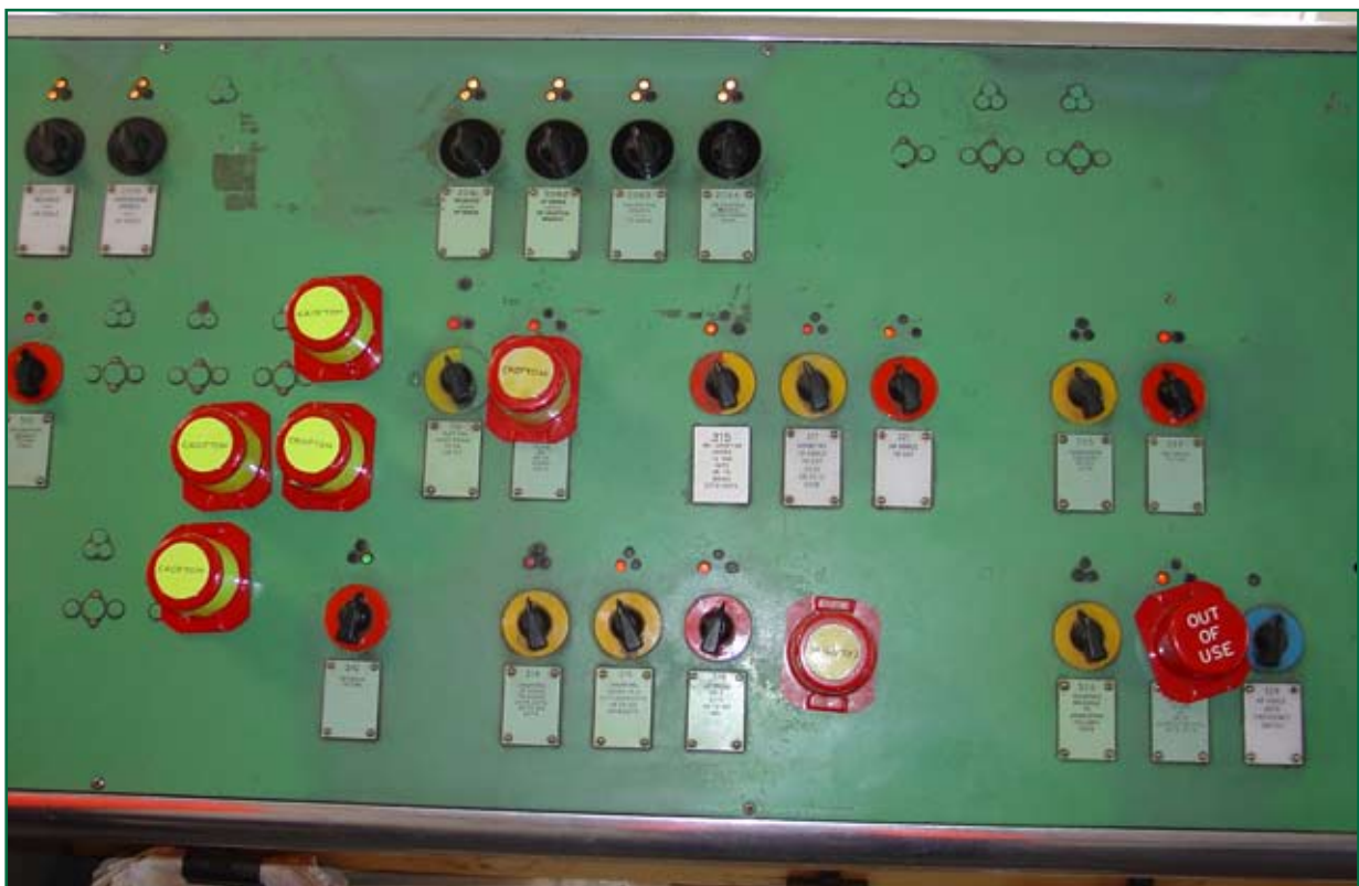
Figure 4: Oakenshaw signal box switch panel showing special crossing reminder appliances
