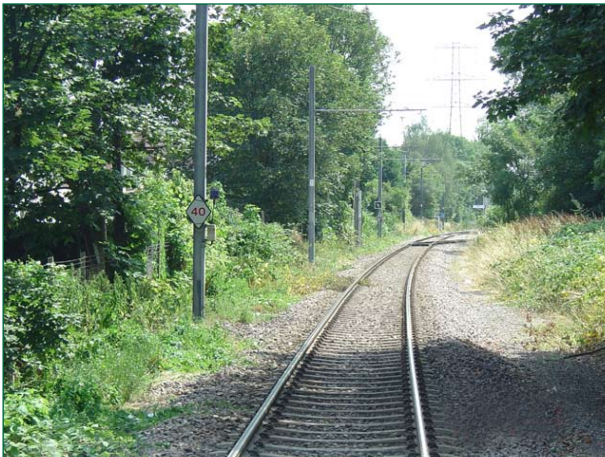
Figure 7: The approach to Phipps Bridge, showing the re-sited speed restriction and the PPI
