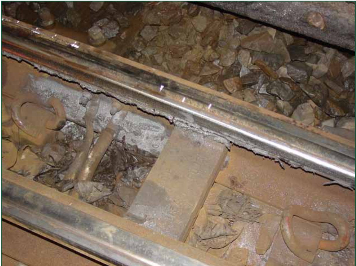
Figure 7: Stock rail near point of derailment, showing sidewear and deposits of powder worn away from rail head
