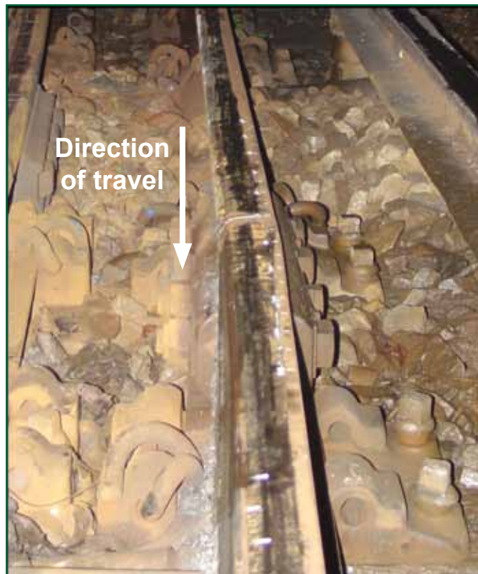
Figure 5: Outer rail at point of derailment, showing misalignment
