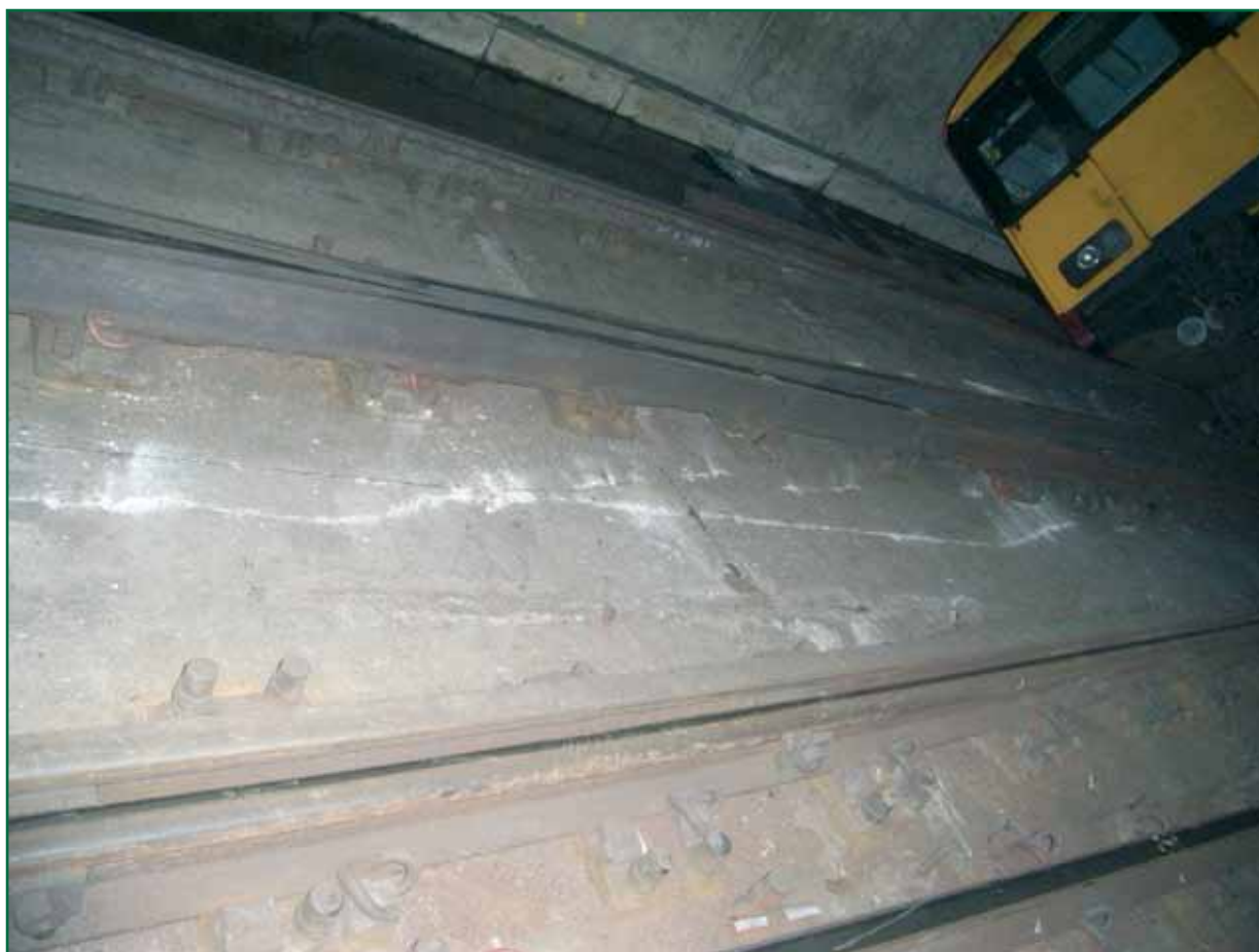
Figure 18: Slab track with fixtures connected directly to the base concrete. Also scores made by the flanges of the derailed wheels.
