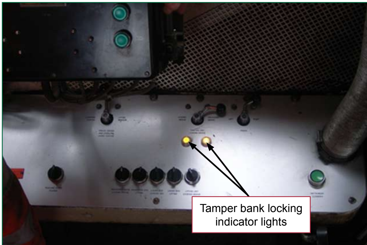
Figure 3: Tamper bank locking indicator lights
