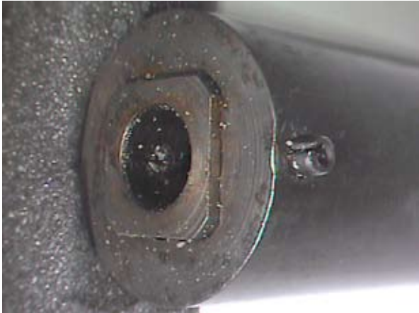
Figure 7: collar showing fractured pin
