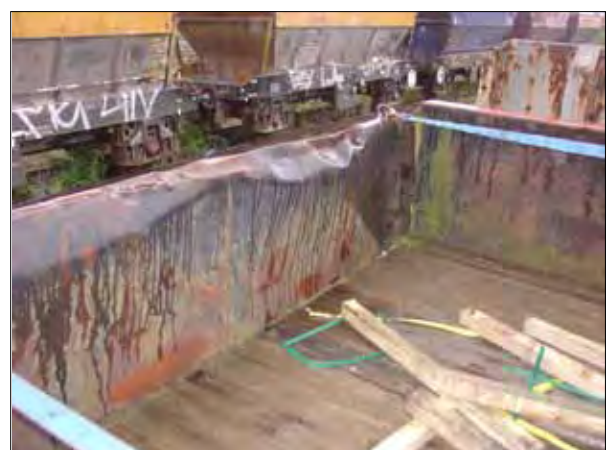
Figure 2: Incident door (held closed by straps) showing damage
