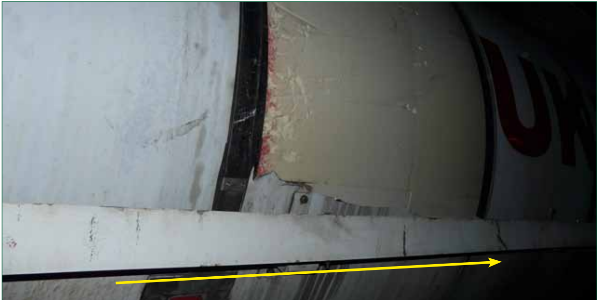
Figure 1: Image of the right-hand side of the tank after the 'H' panel cladding section had been cut off at Carstairs (direction of travel indicated with yellow line)
