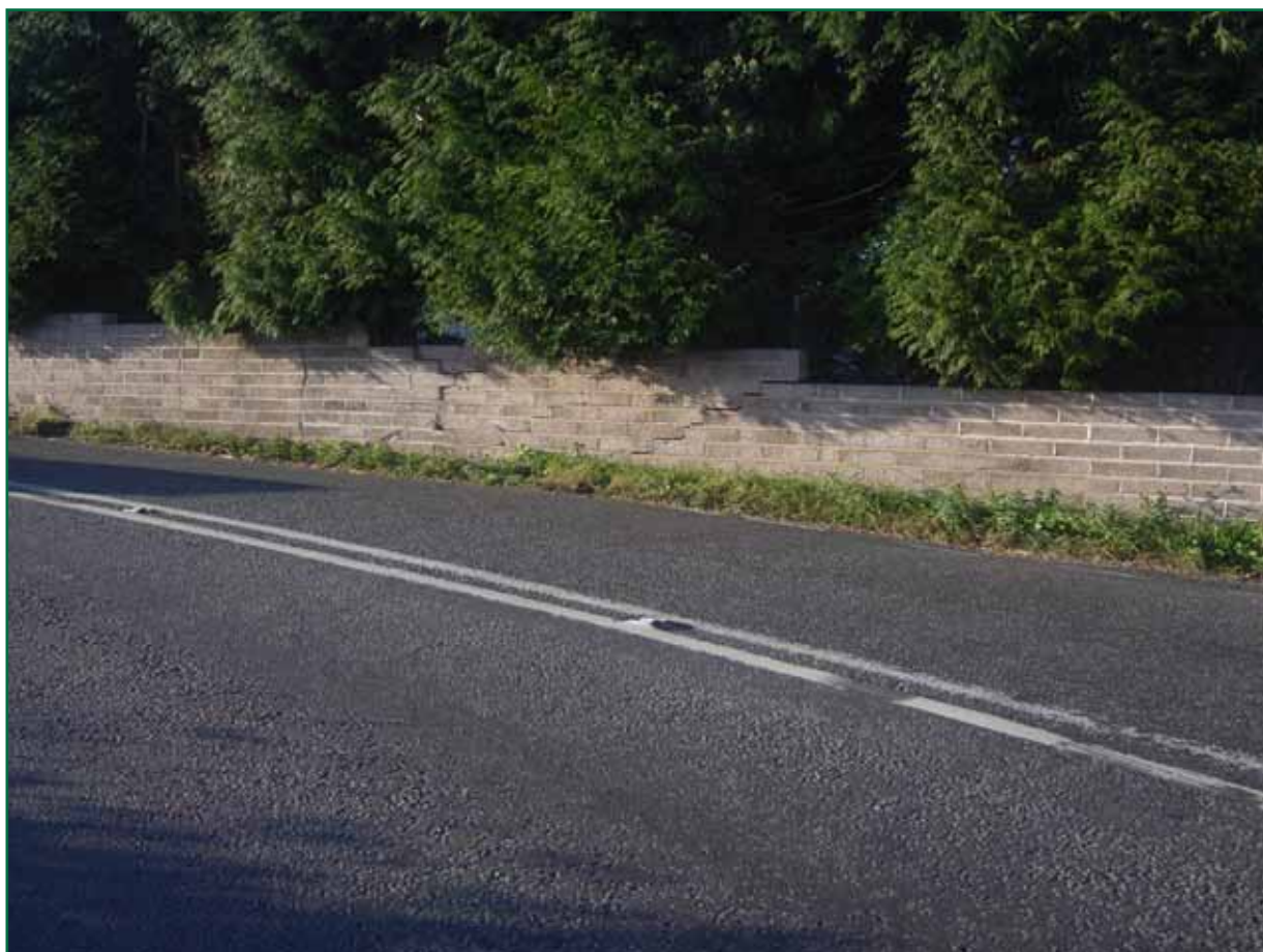
Figure 2: Concrete block wall showing impact damage
