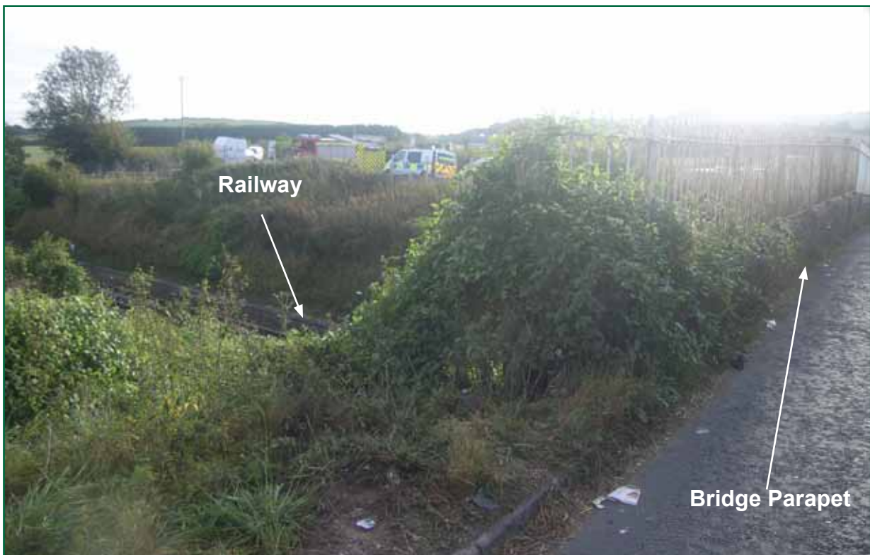
Figure 4: Gap at north-west corner of the bridge through which the car travelled
