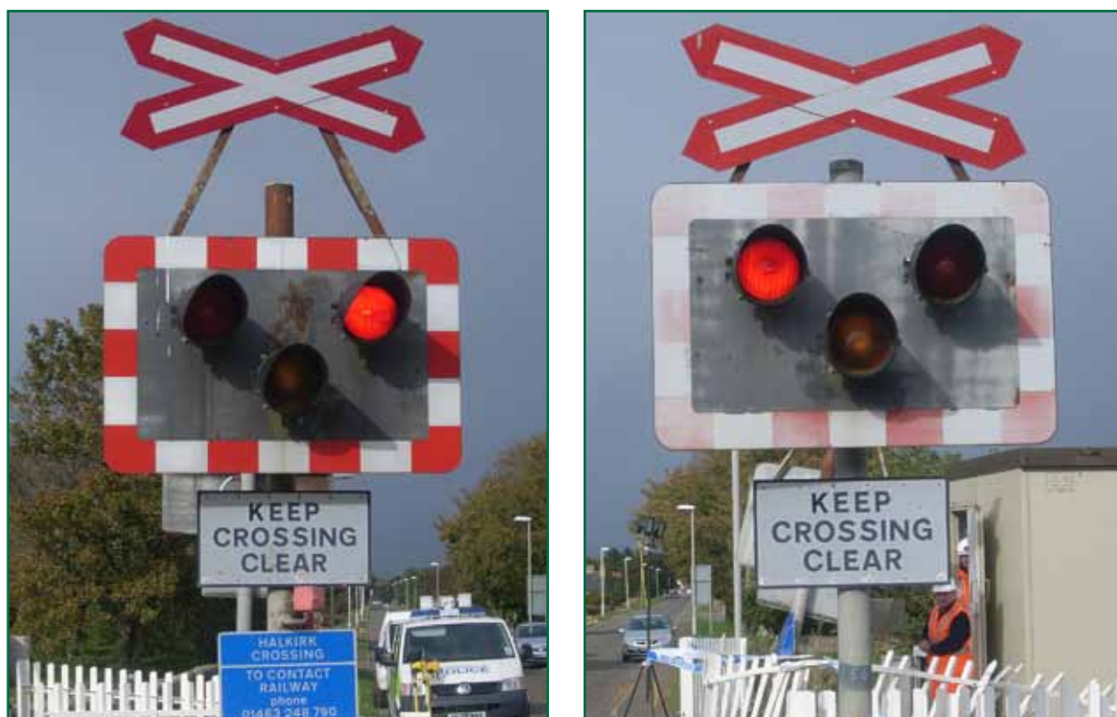
Figure 7: Condition of road traffic light signals, Halkirk crossing, south side
