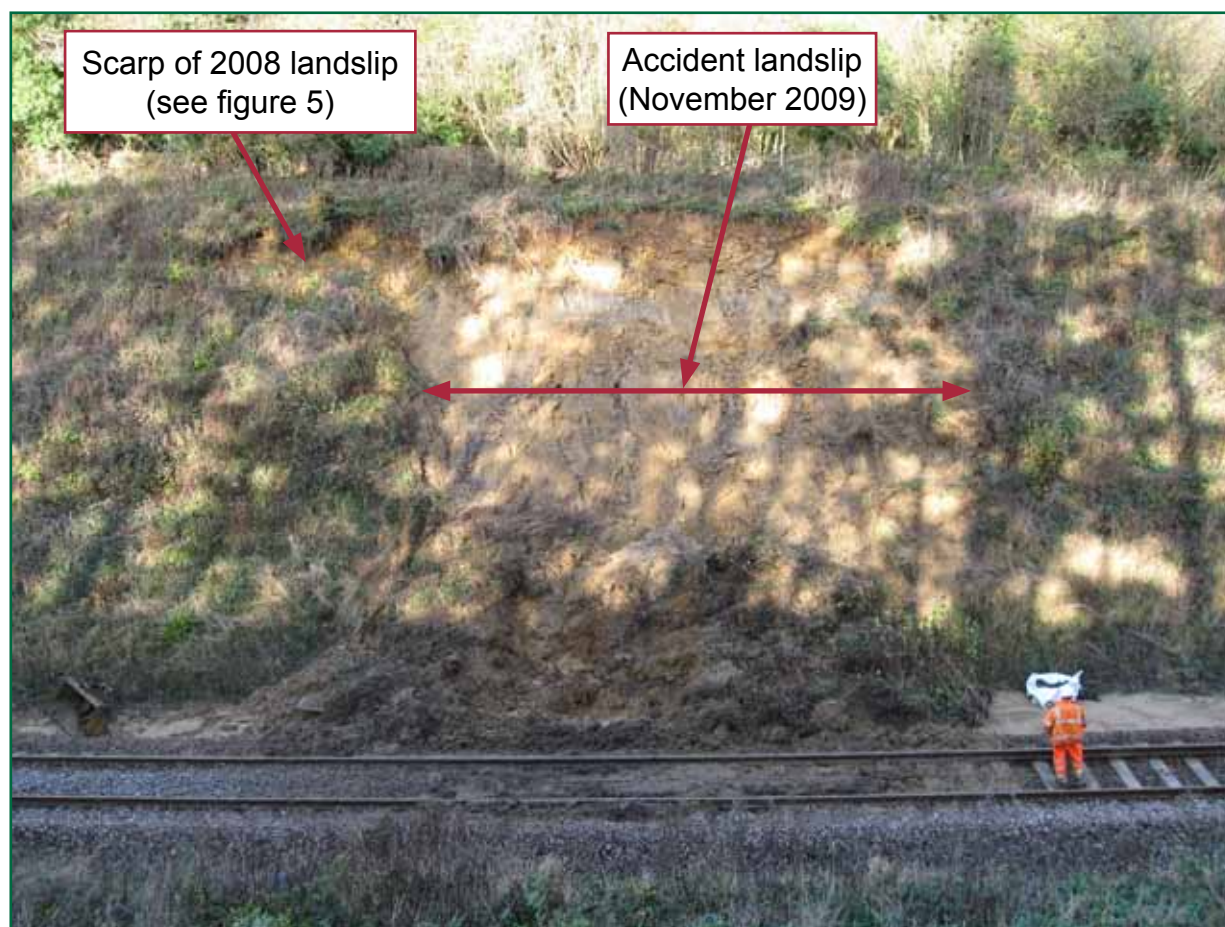
Figure 6: Accident and December 2008 landslips (Image courtesy of Network Rail)
