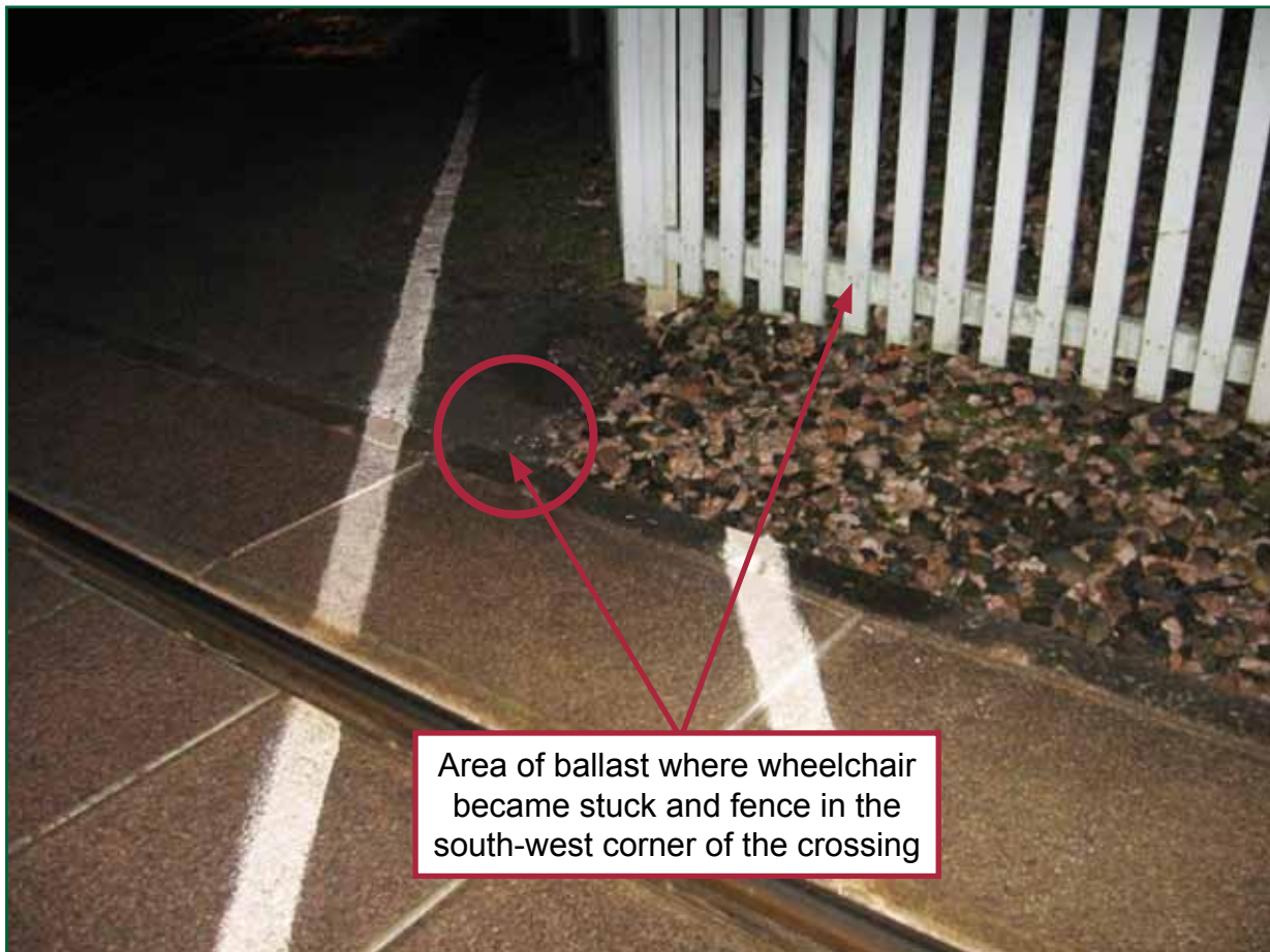
Figure 2: Area of ballast and fence in south-west corner of the crossing (photograph courtesy of Network Rail)
