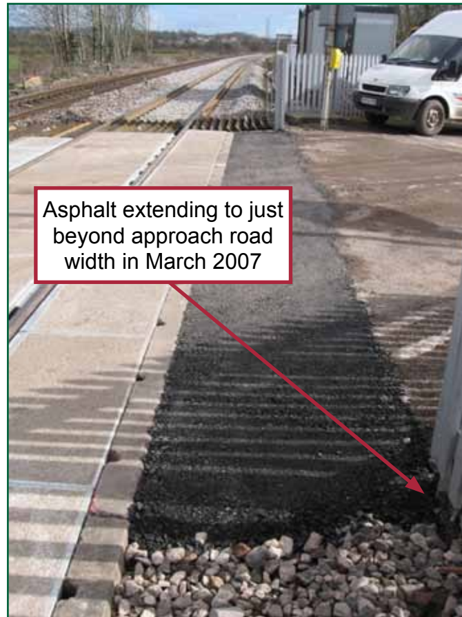
Figure 10: The asphalt section following the work in March 2007 (photograph courtesy of Network Rail)
