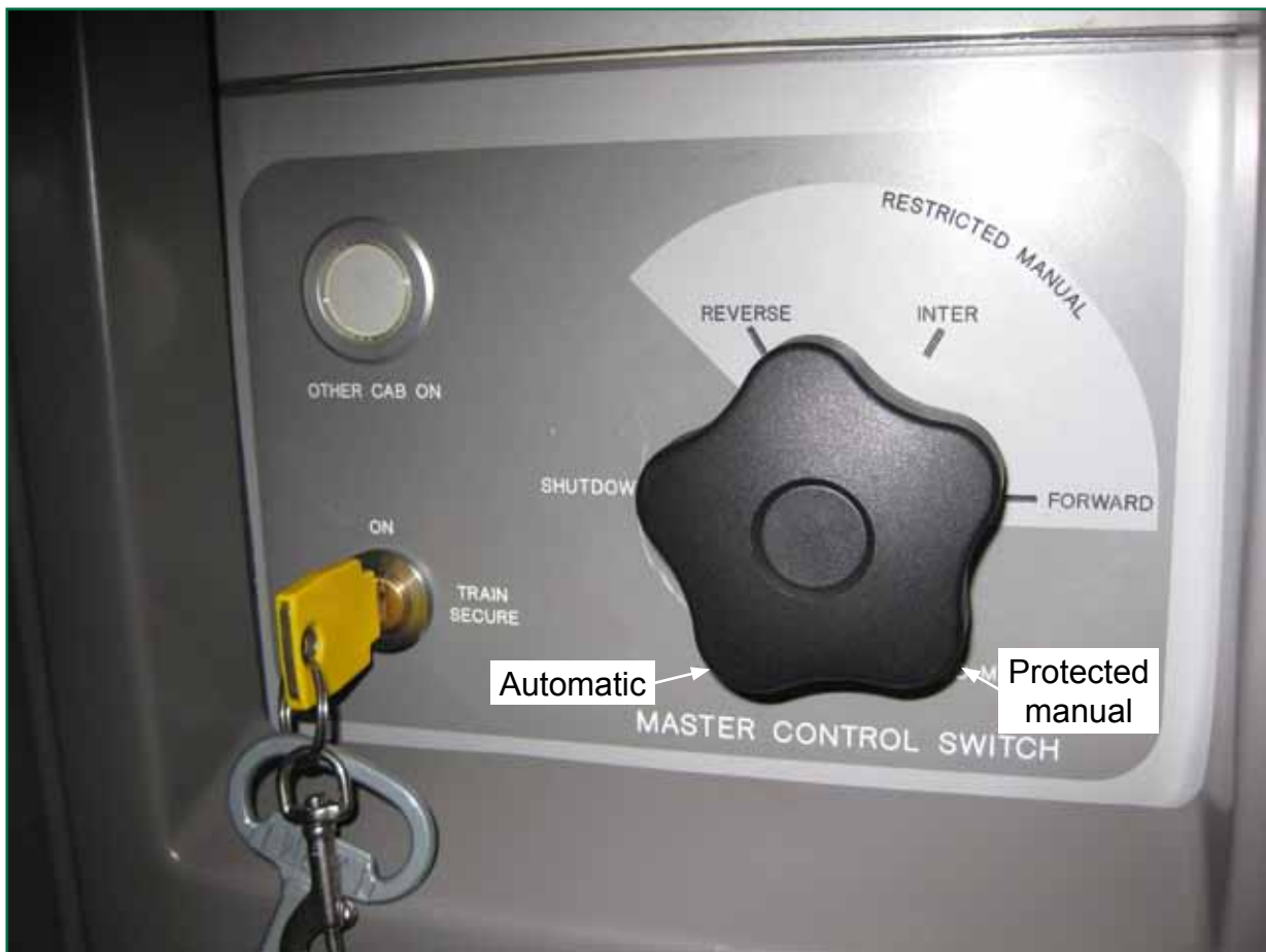
Figure 4: Master control switch 2009 tube stock
