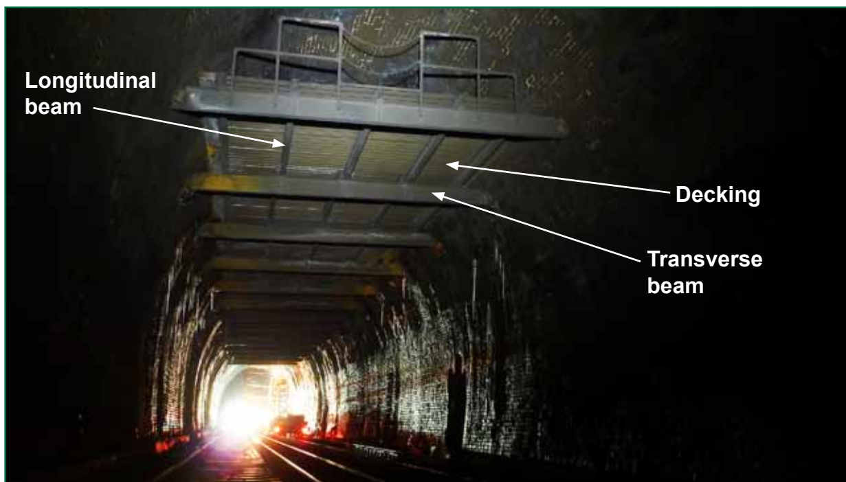
Figure 2: Water catchment tray structure
