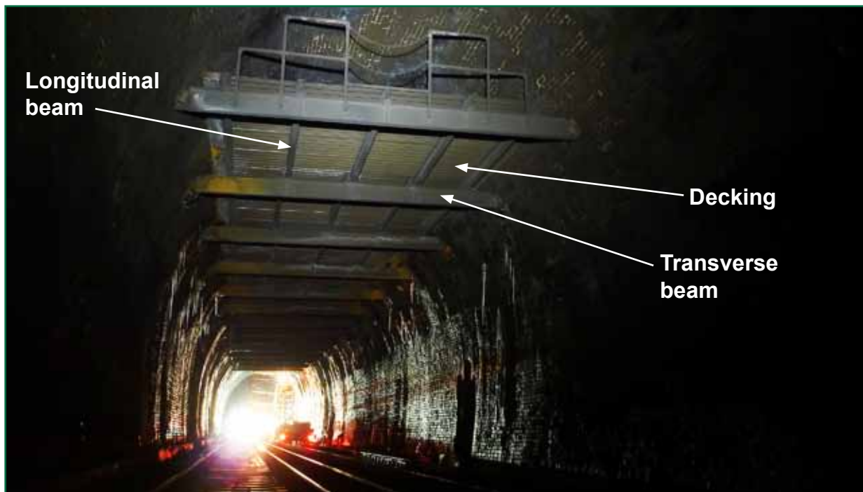
Figure 2: Water catchment tray structure
