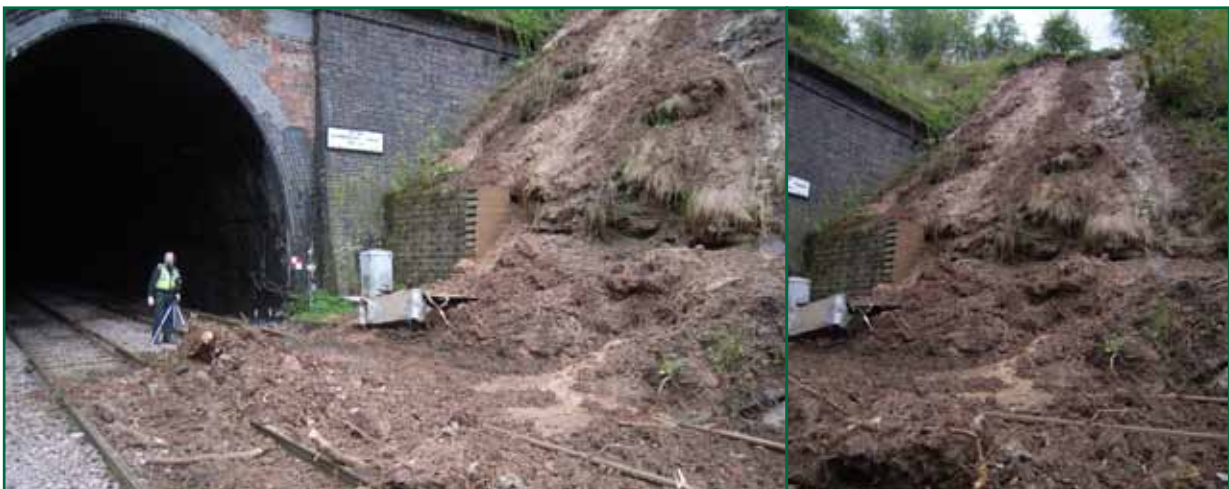
Figure 1: The landslip outside Clarborough Tunnel
