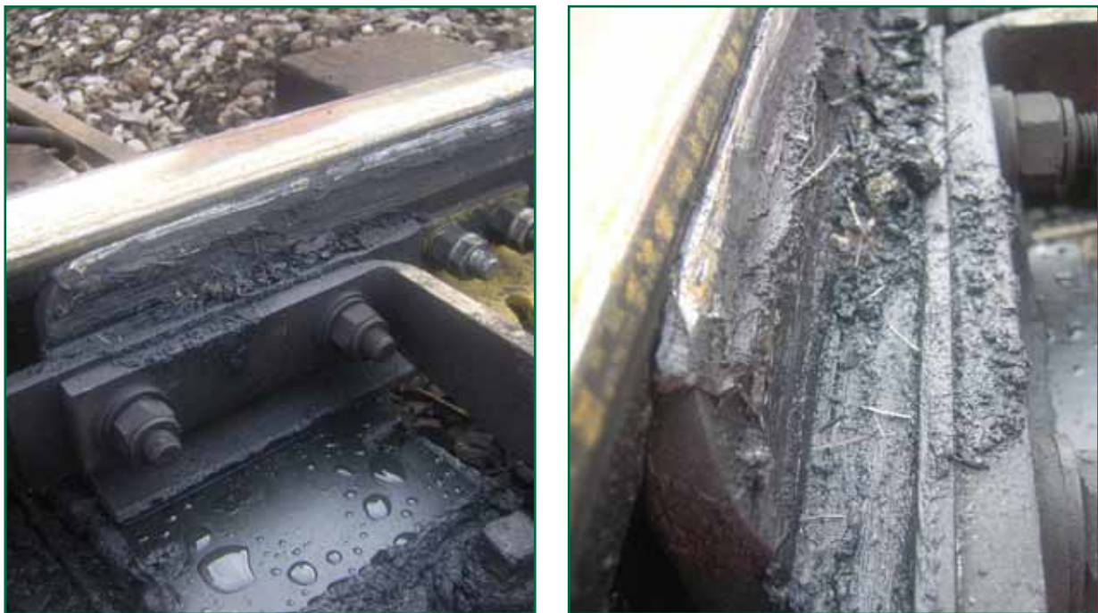
Figure 9: Left-hand switch rail at No.75 points immediately after derailment
