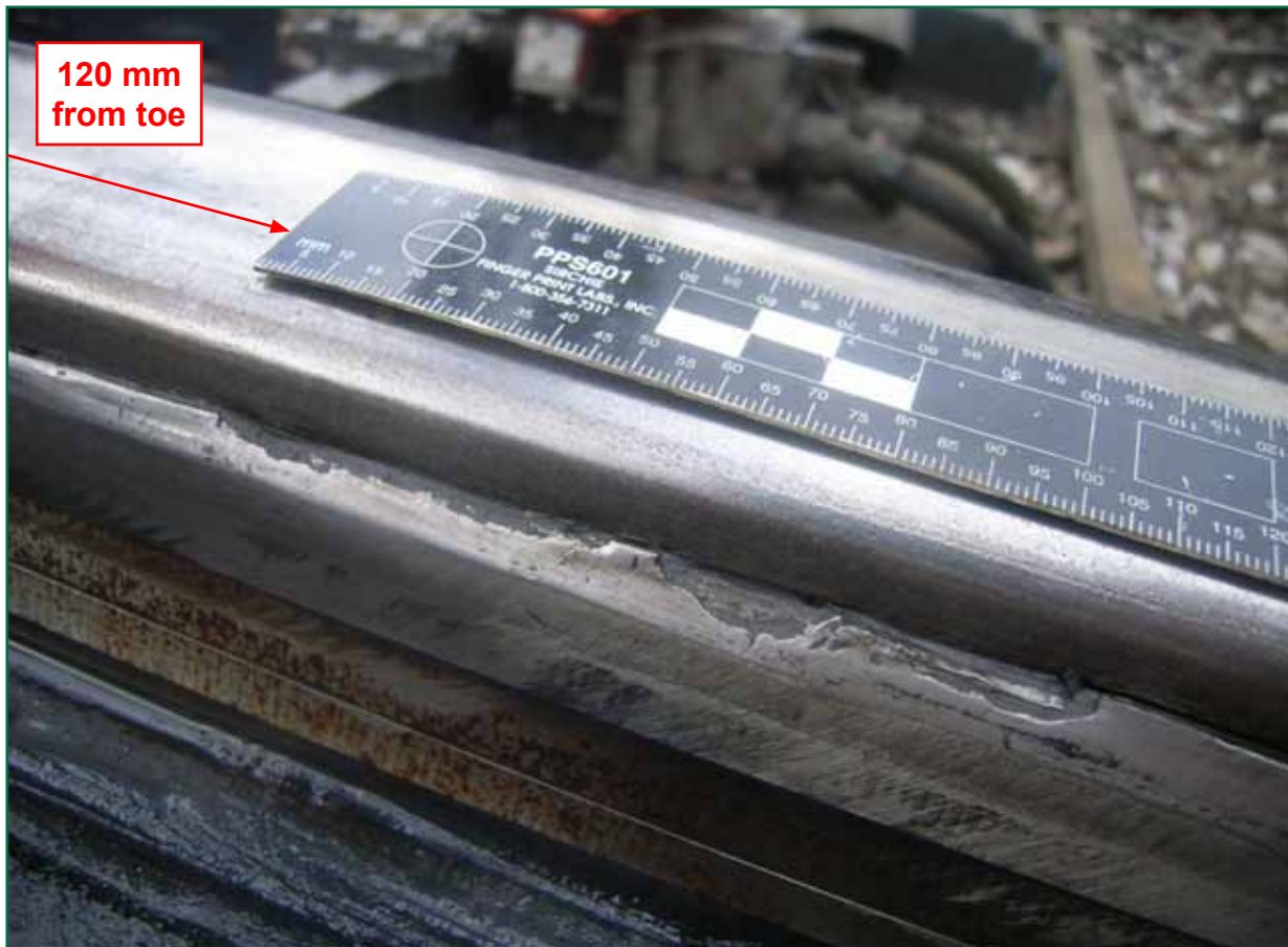
Figure 7: Left-hand switch rail damage
