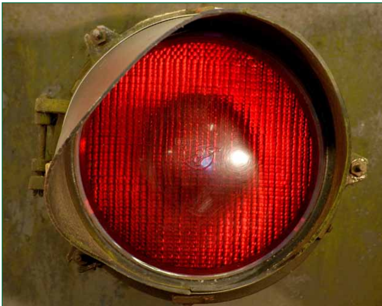
Figure 5: Close up of 'Bliss' lens fitted to one of the wig-wag units at the north side of the crossing
