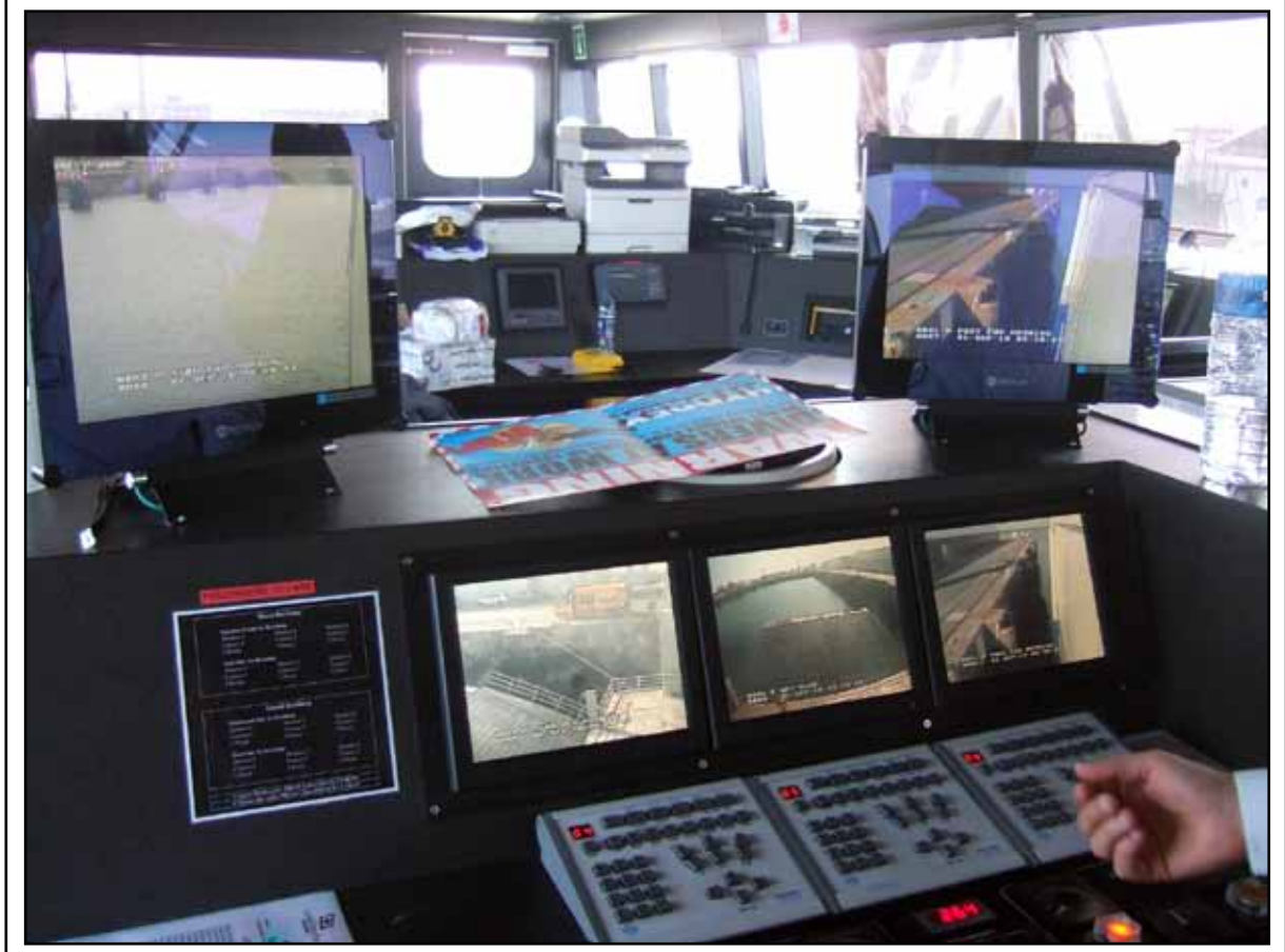
CCTV monitors from different heights of eye
