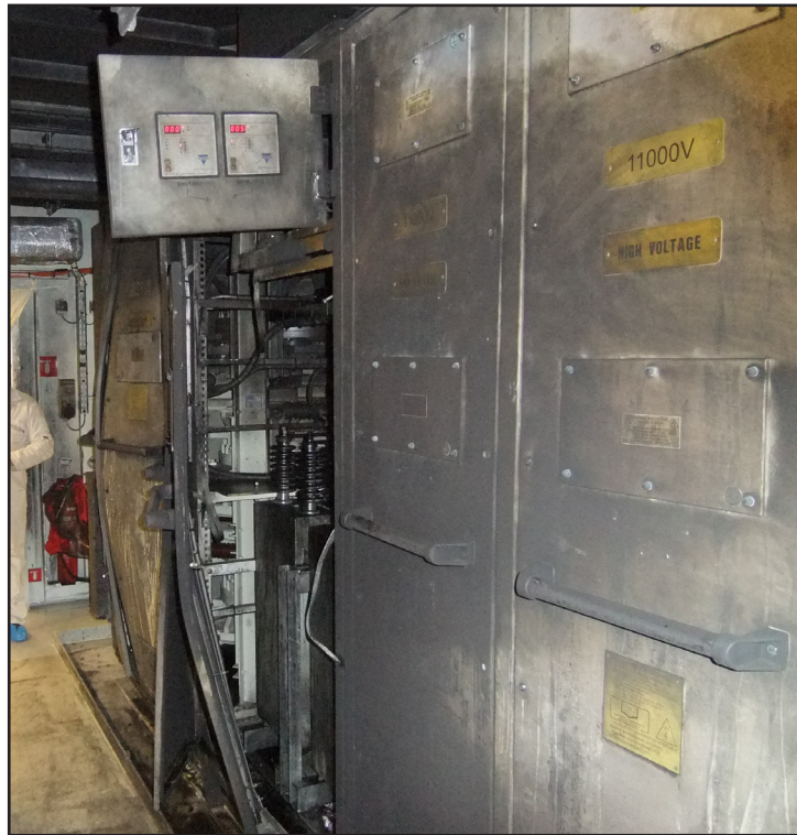
Soot staining on the blown-out doors of the harmonic filter casing
