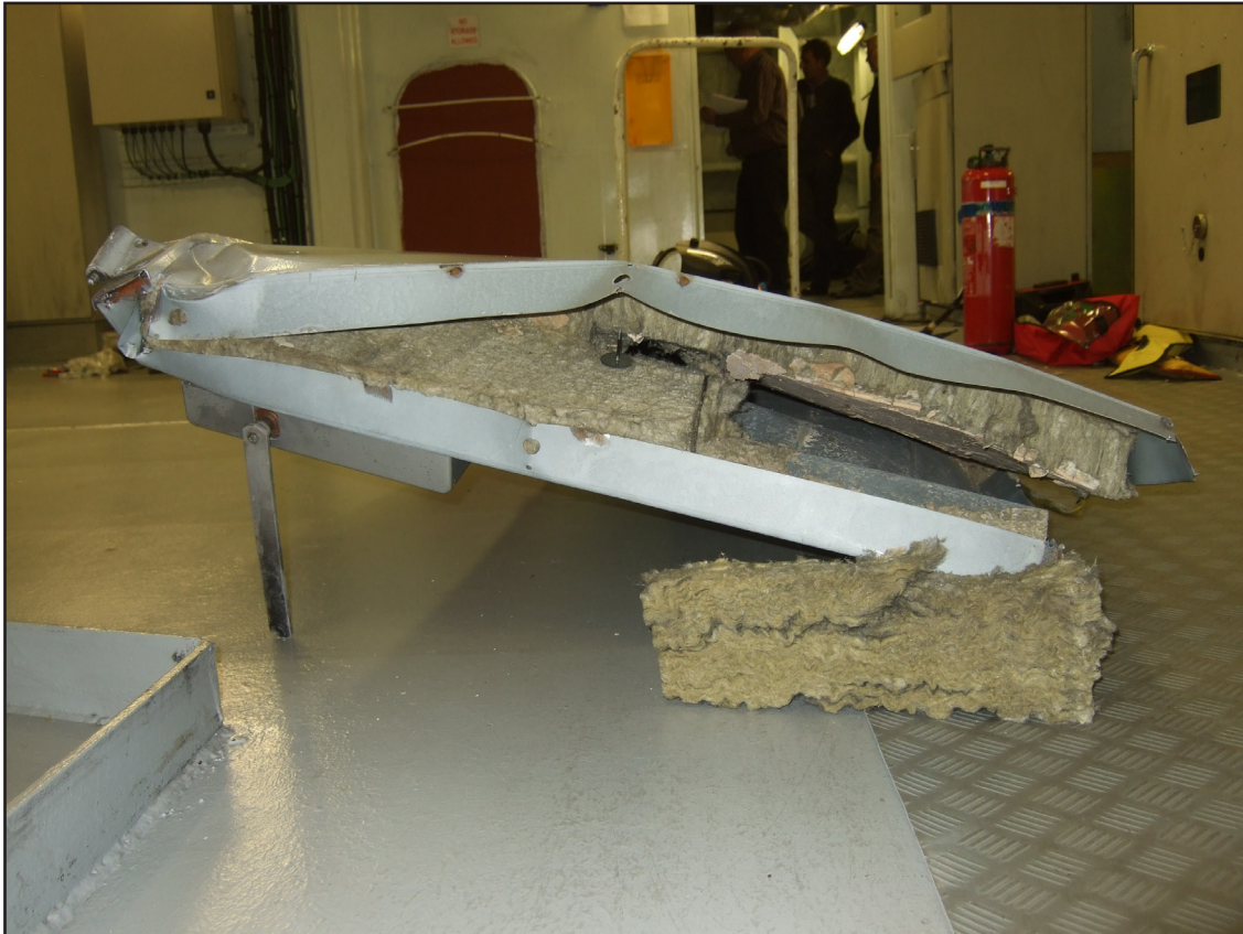
Damaged steel door to the harmonic filter compartment
