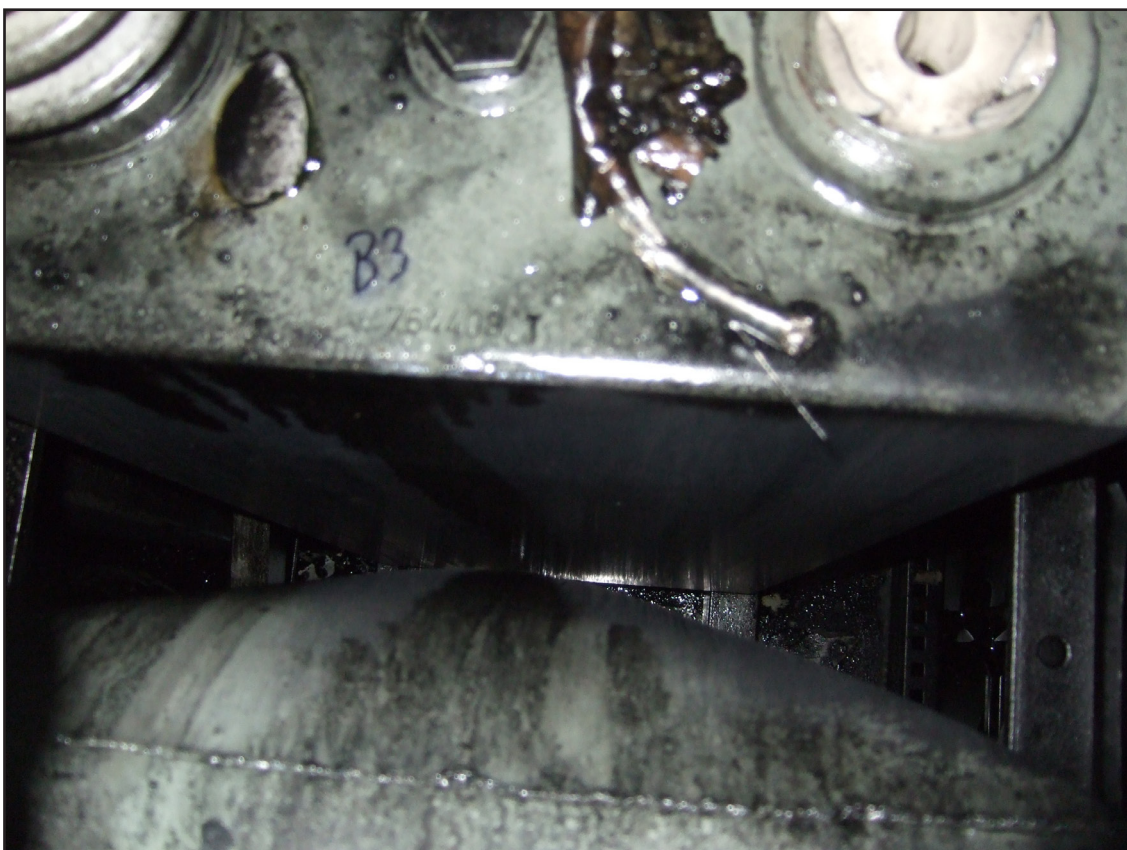
Top view of two capacitors indicating one which had developed a severe bulge due to internal pressurisation
