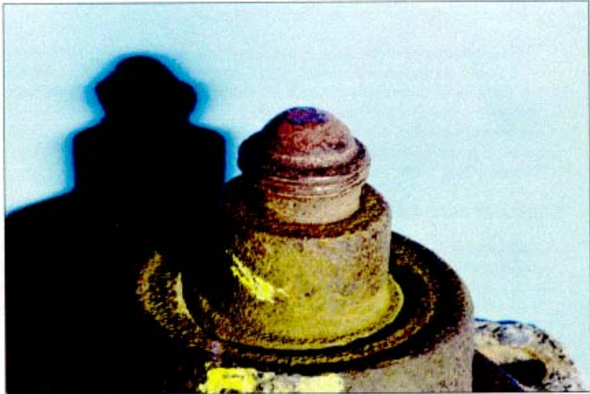
Figure 23 - Aft side valve spindle, showing worn or stripped cap retaining threads
