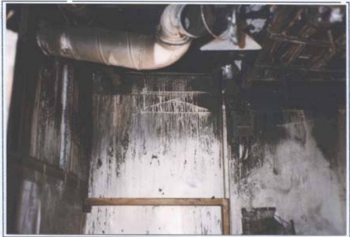
Fig 4 General view of smoke and water damage to upper parts of electrical locker bulkhead. Note evidence of fire in void space only.
