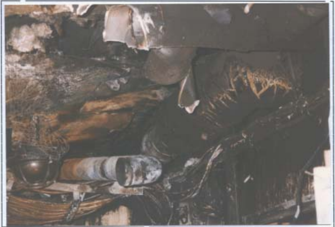
Fig 3 General view of fire and water damage to ventilation trunking and insulation.
