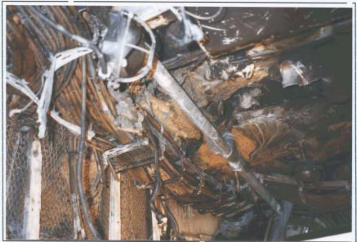
Fig 2 Close up view of damaged electrical cabling and deckhead insulation.
