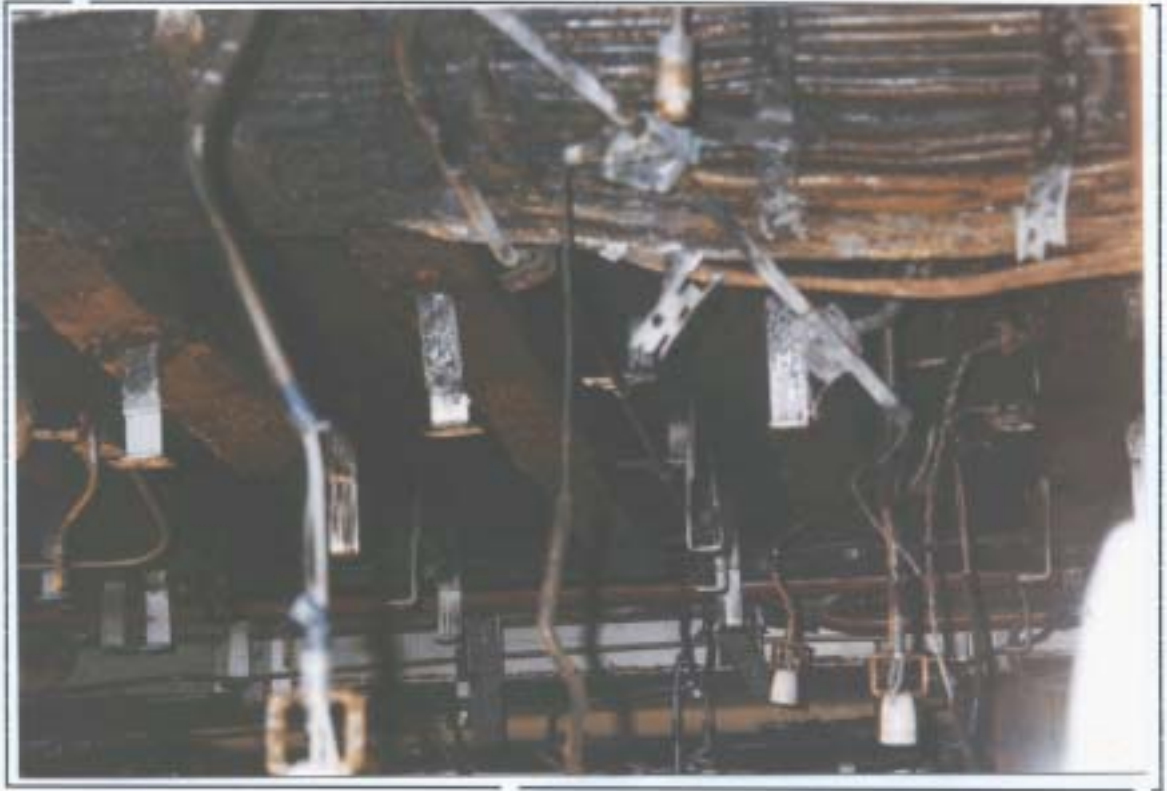
Fig 1 General view of fire and water damage to electrical locker deckhead.
