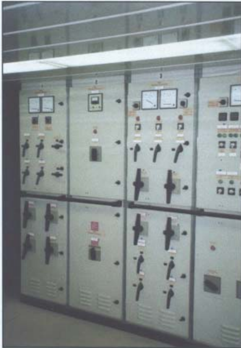
Main Switchboard (Port Side) Panels 1, 2 & 3
