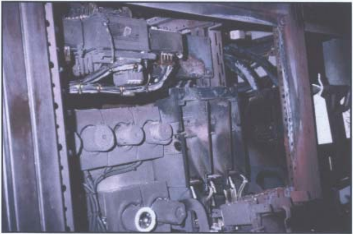
Car Deck Ventilation Fan Fuse Switch. Note arcing damage to top of Fuse Switch (incoming power).
