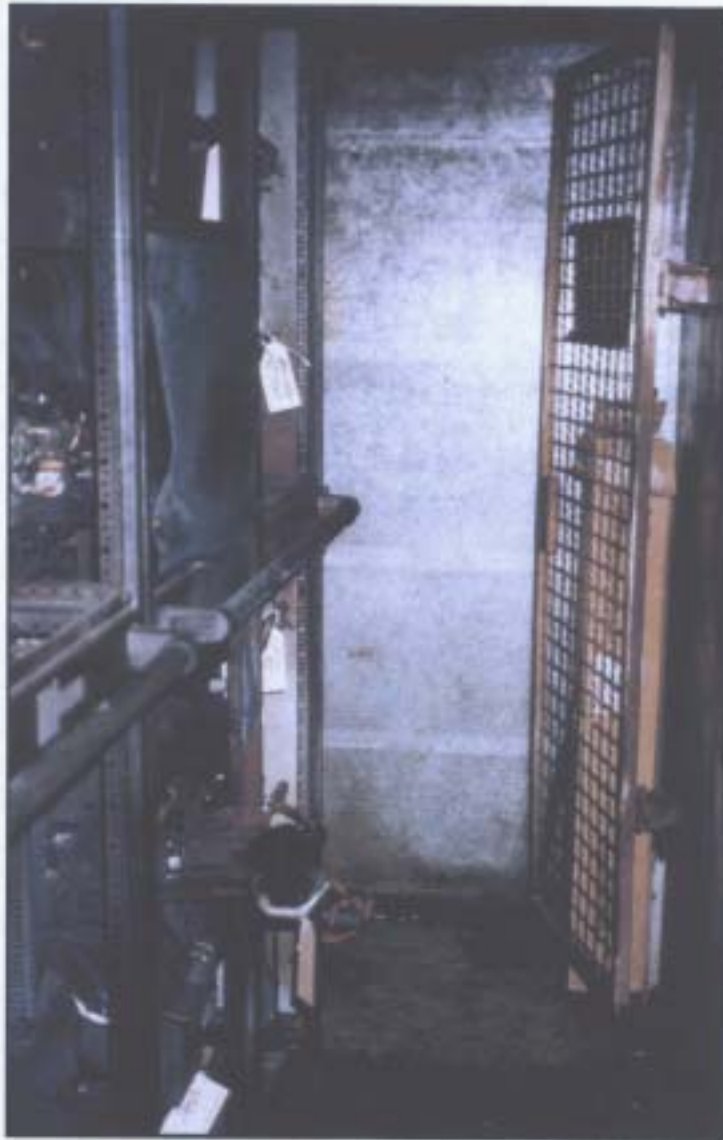
Port side entrance to rear of Main Switchboard. Note open Fuse Switch for Car Deck Ventilation Fans
