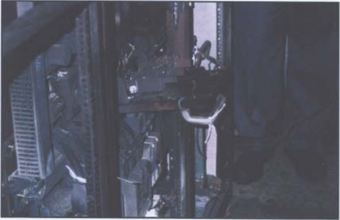
Open Fuse Switch for Car Deck Ventilation with Fuse in situ
