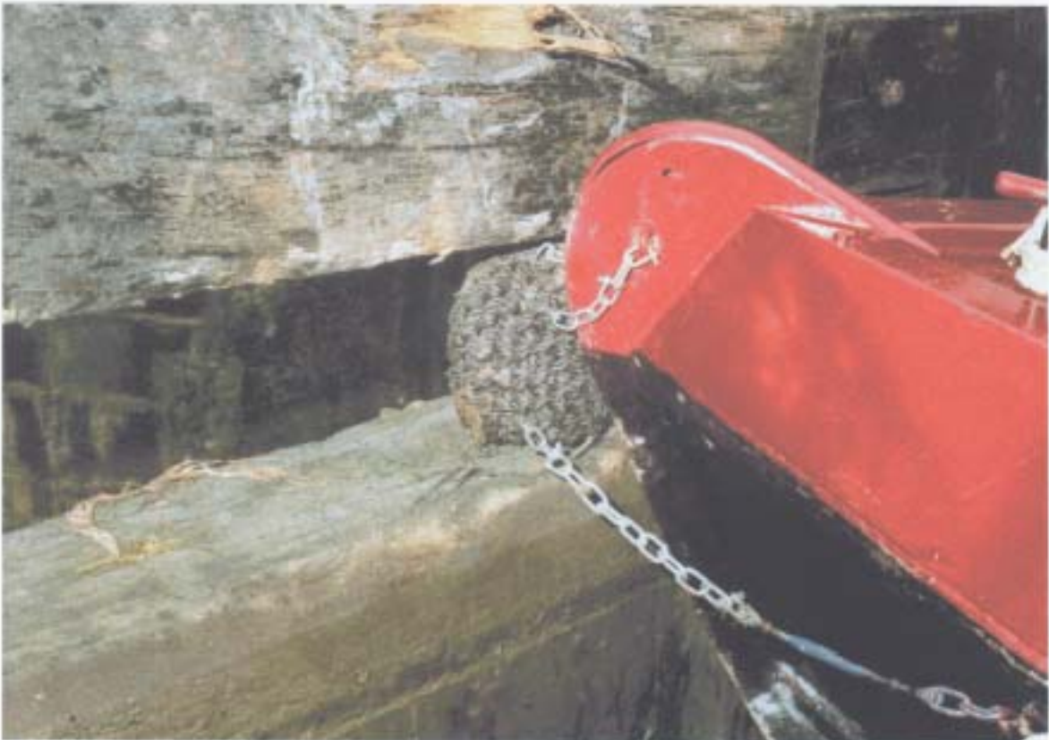
The water level in the lock was dropped and the fender was allowed to become caught in the gap between the balance beam (top) and the top of the gate (below).
