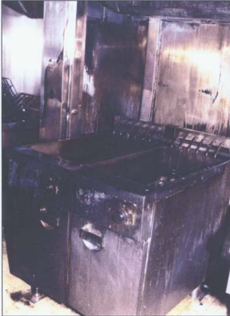
Figure 4. The coupled deep fat fryers. The unit on the left is the aft unit in which the fire occurred.
