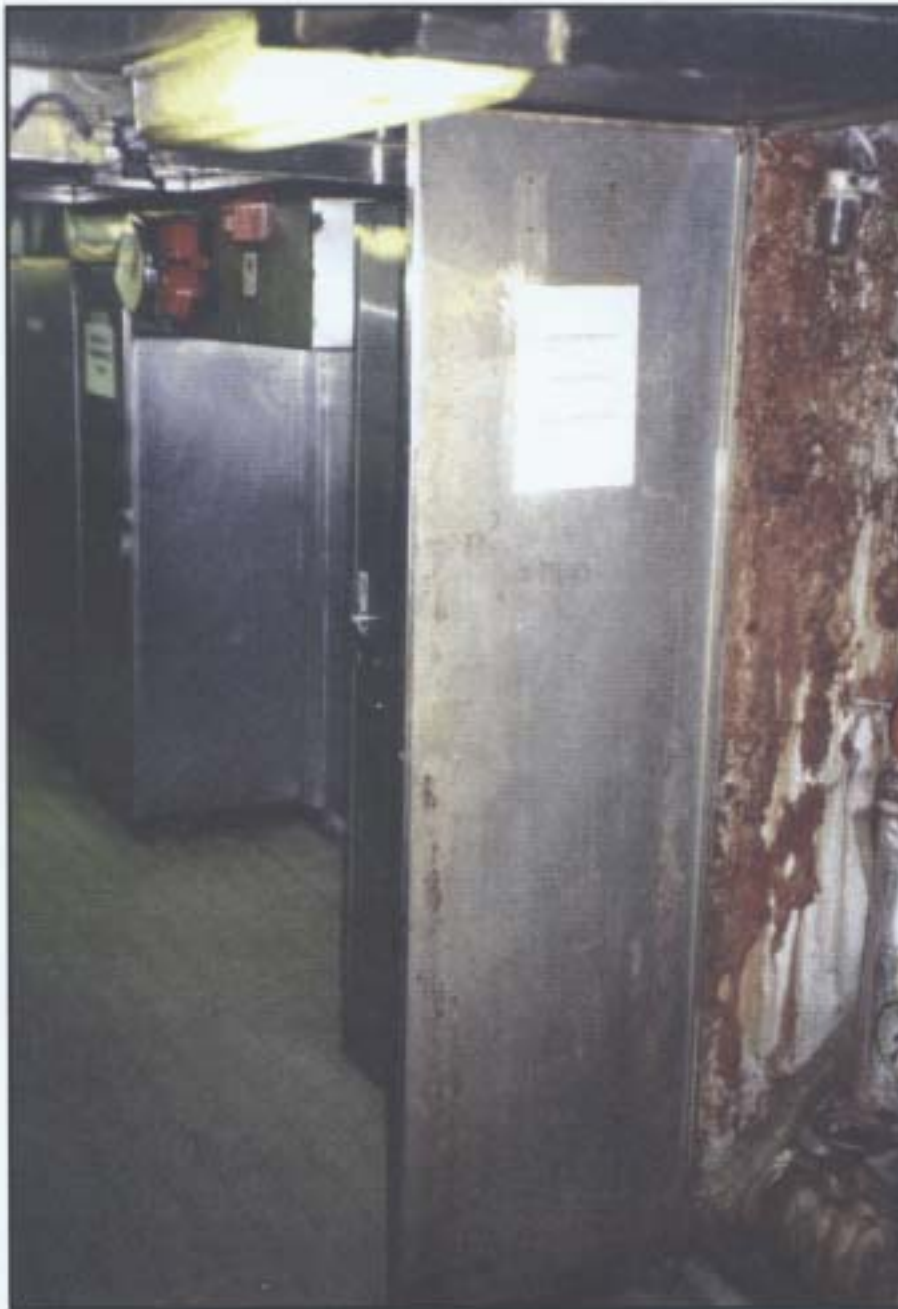
Figure 9. Control cabinet for steam smothering system to left of picture. Working passage within galley leading off to the right.
