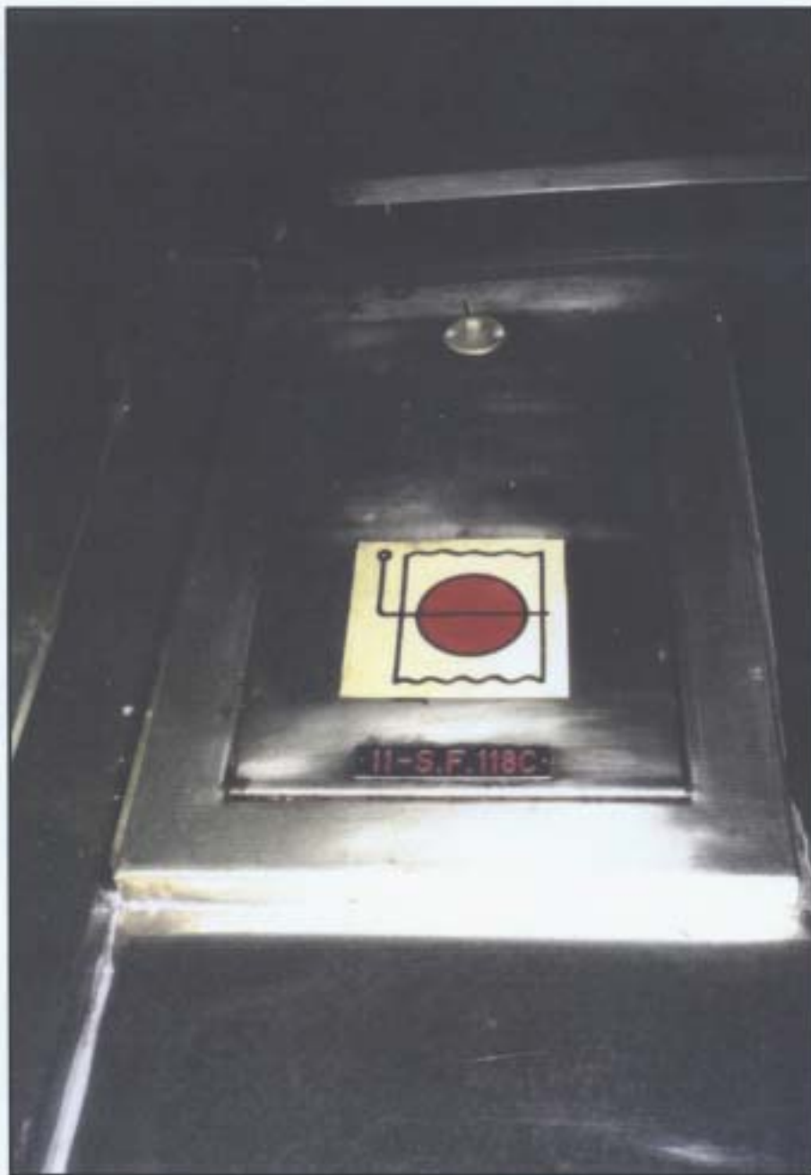
Figure 8. A galley damper cover, with label.
