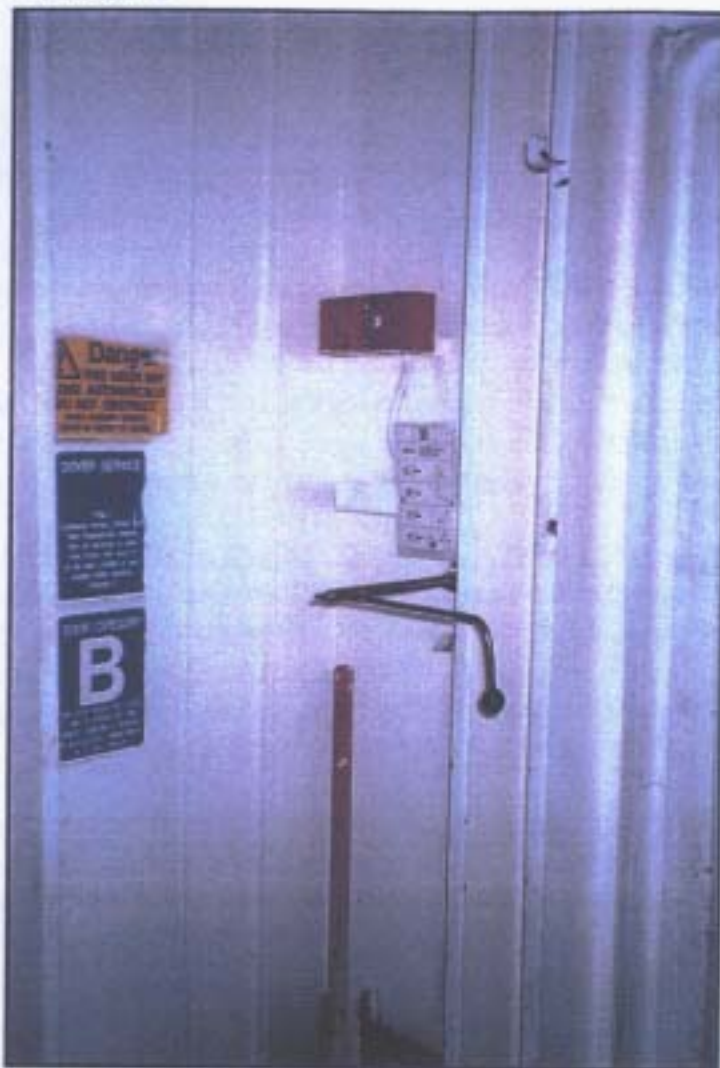
"Cranked" operating lever on separator room side of watertight door No.6.
