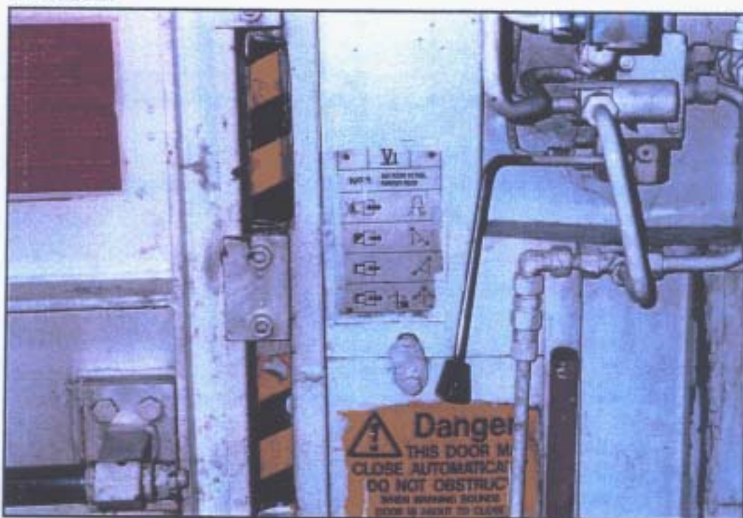
"Cranked" operating lever on generator room side of watertight door No.6.
