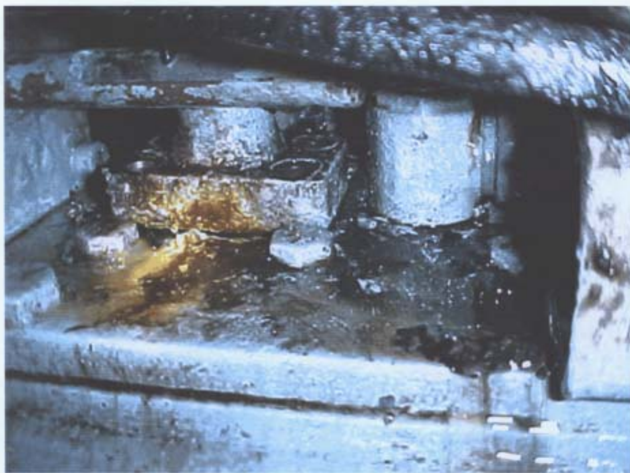
Close up of leaking HP flange connection (bolts removed)
