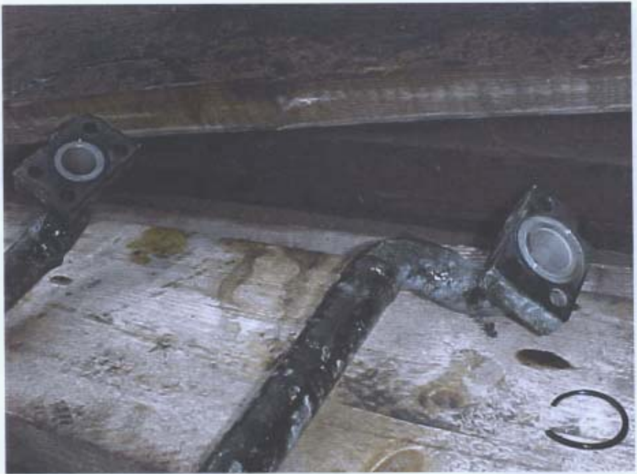
General view of pipe flange connections
