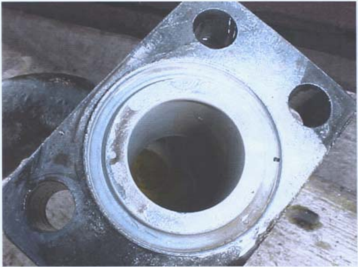
Undamaged seal ring groove on pipe flange
