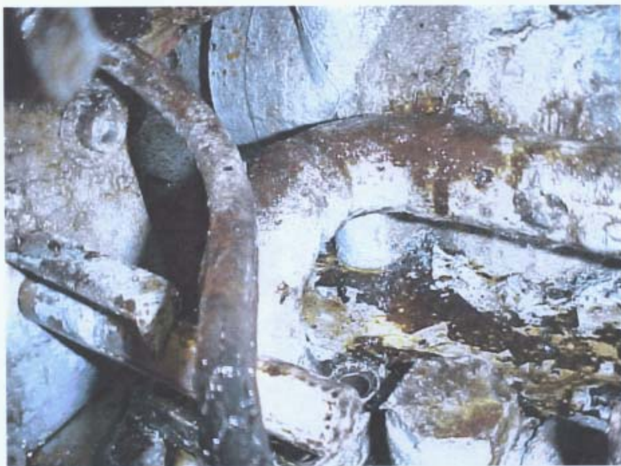
Close up view of O/D box after fire
