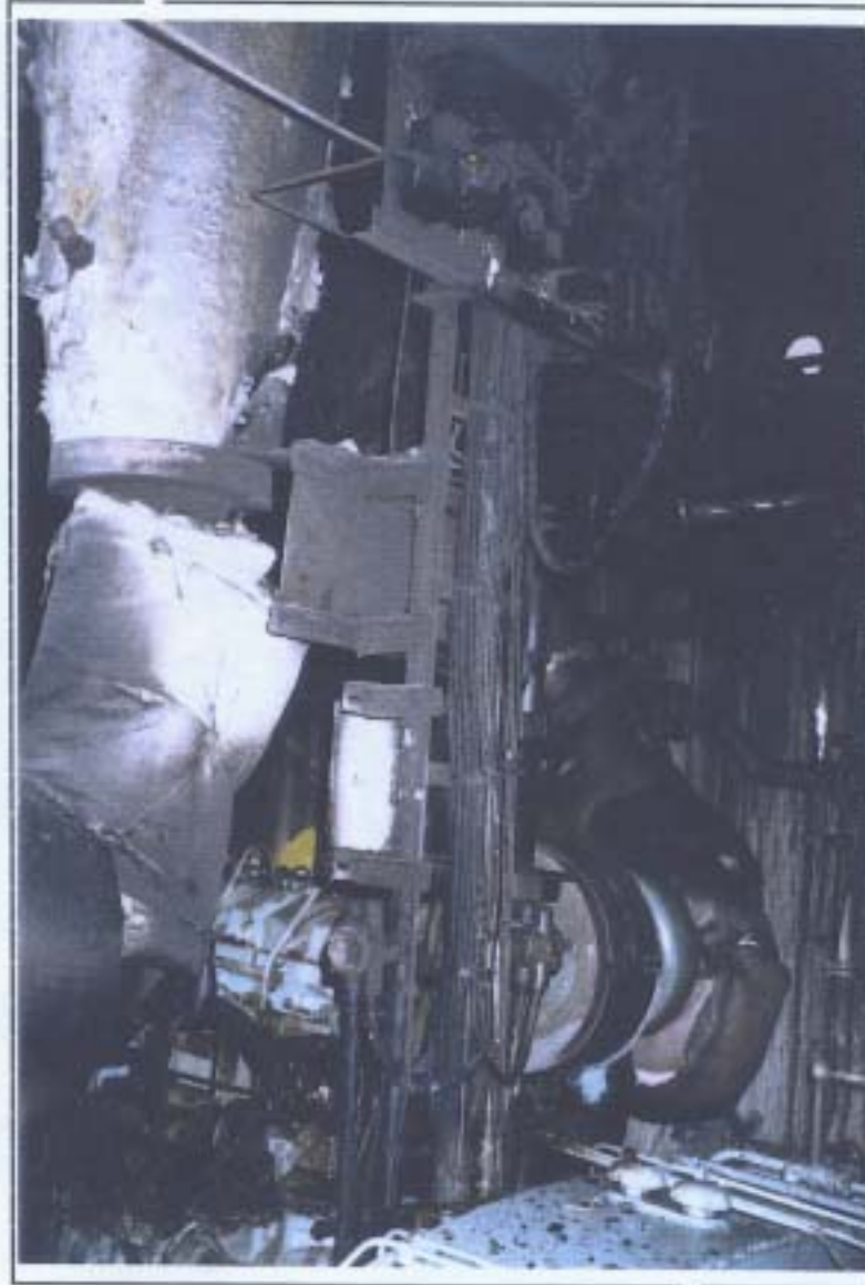
Fig 7 View of alarm and signal actuator panel above starboard gear box showing increasing damage towards the deckhead.
