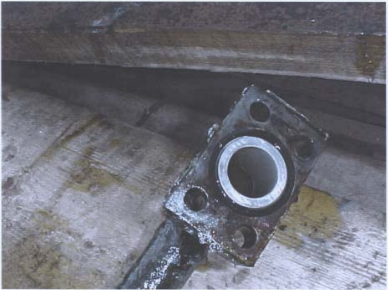
Other pipe flange showing seal ring complete and in place
