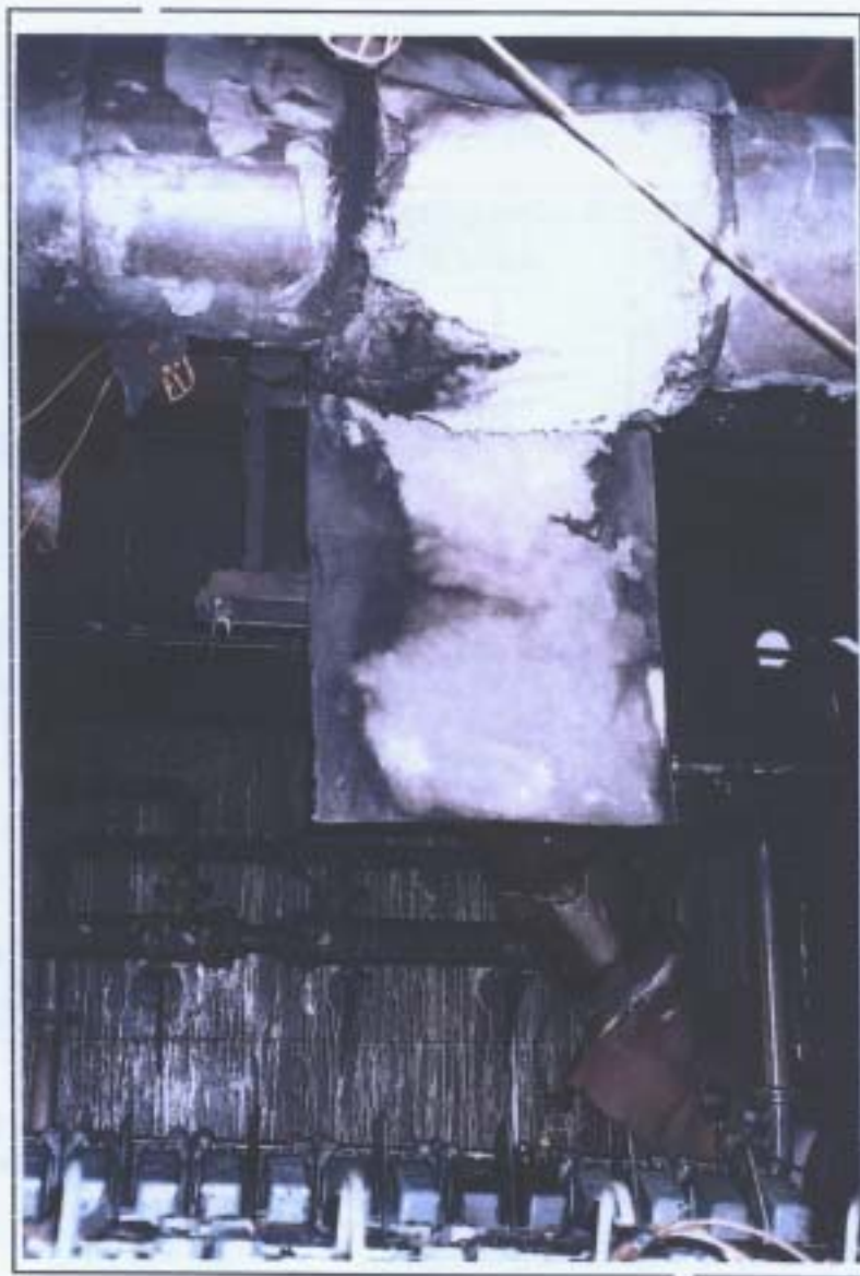
Fig 9 View of starboard side deckhead and bulkhead interface showing soot and oil runs as well as failure of lagging clips.
