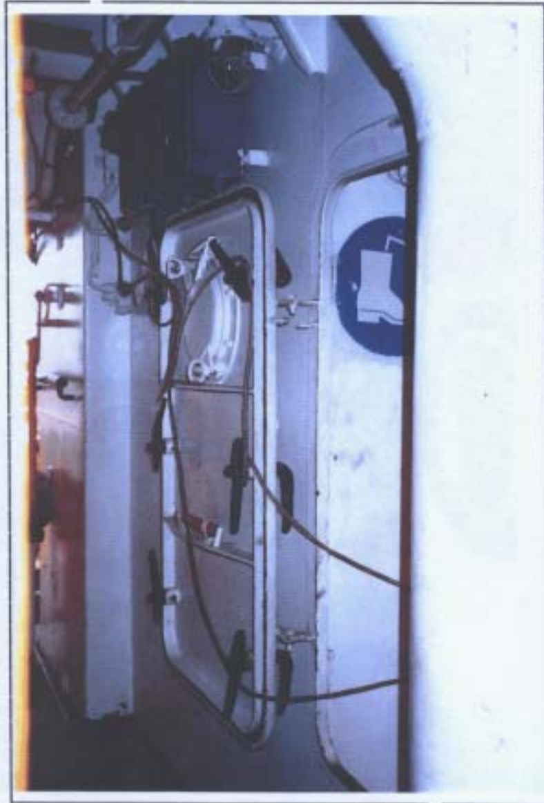
Fig 12 View looking aft through port alleyway showing outer engine door flat against funnel casing. This is not as shown on GA.
