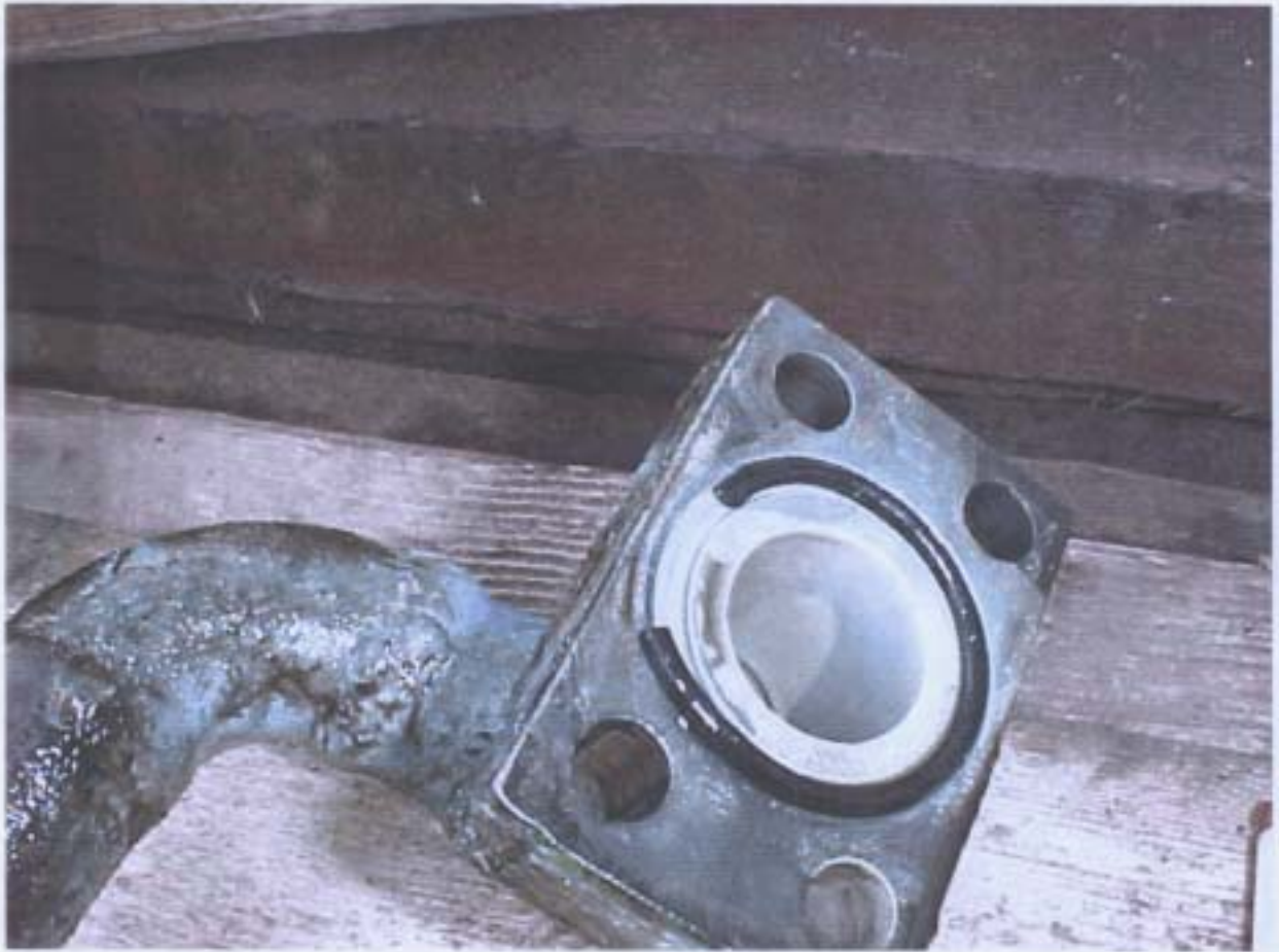
Pipe flange showing missing section of seal ring
