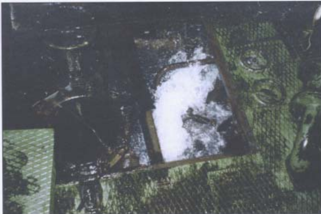
General view of inlet pipe showing S.W. pipe leaking even with temporary seal fitted externally
