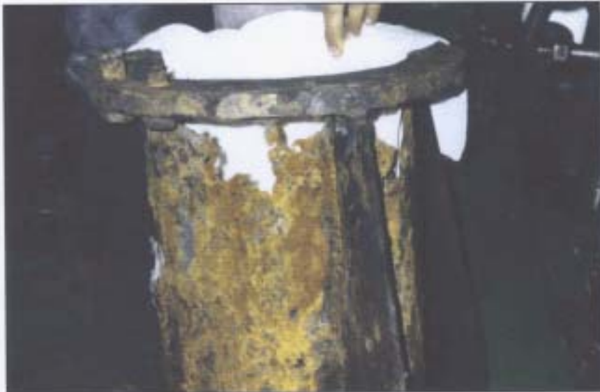
Extent of corrosion
