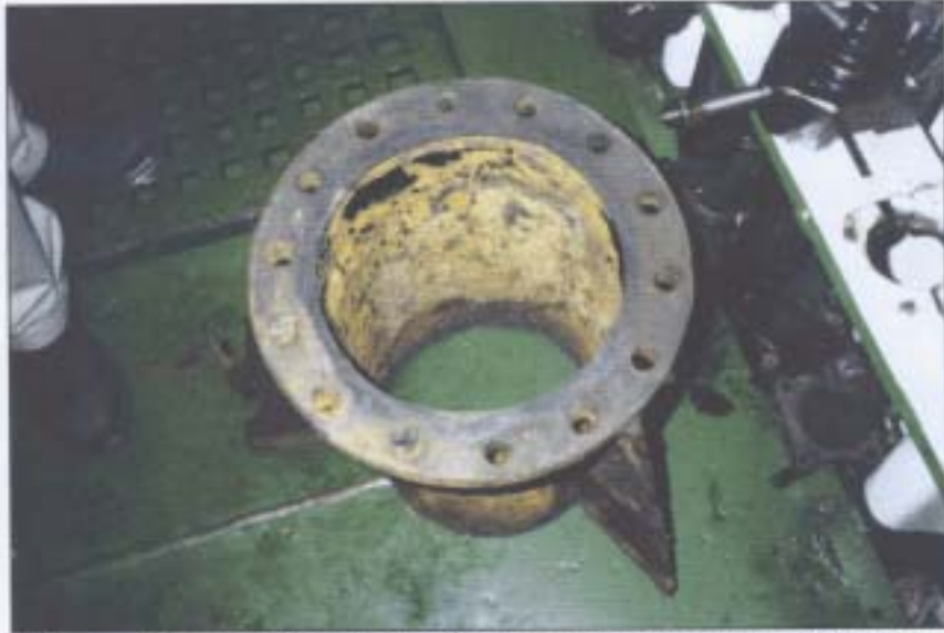
General view of pipe after being removed from top of sea chest
