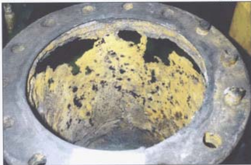
Extent of corrosion on sea inlet pipe. Isolating valve sat on flange.
