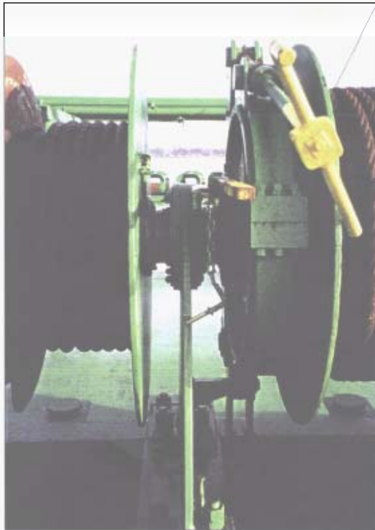
The deck-mooring winch showing the brake and clutch mechanism
