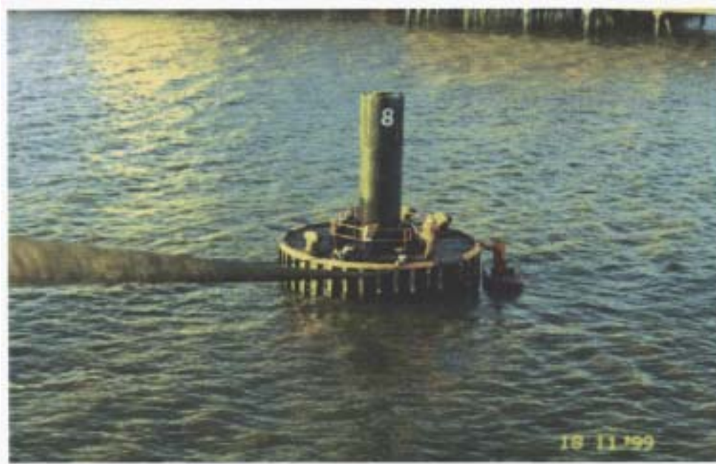
A view of dolphin No 8 taken from Alfa Britannia showing the two breast lines
