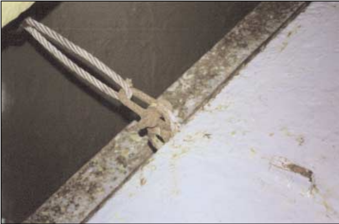
Leading edge of hatch cover showing wire, shackle, and butt of old eye
