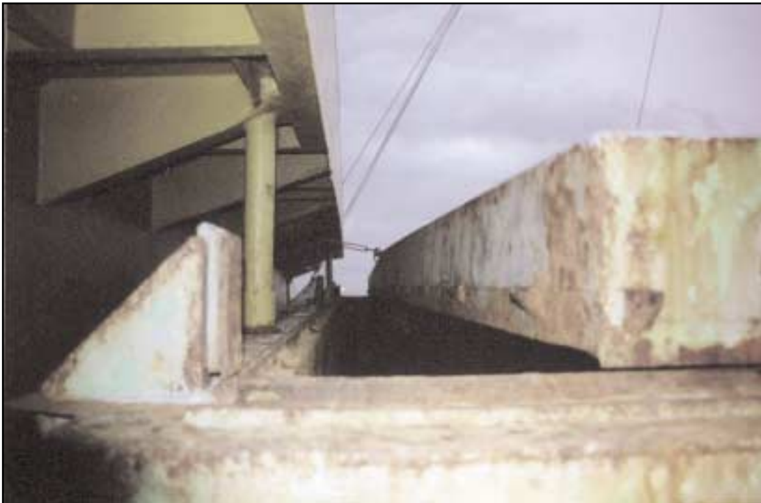
Leading hatch cover in approximate position at the time of the accident
