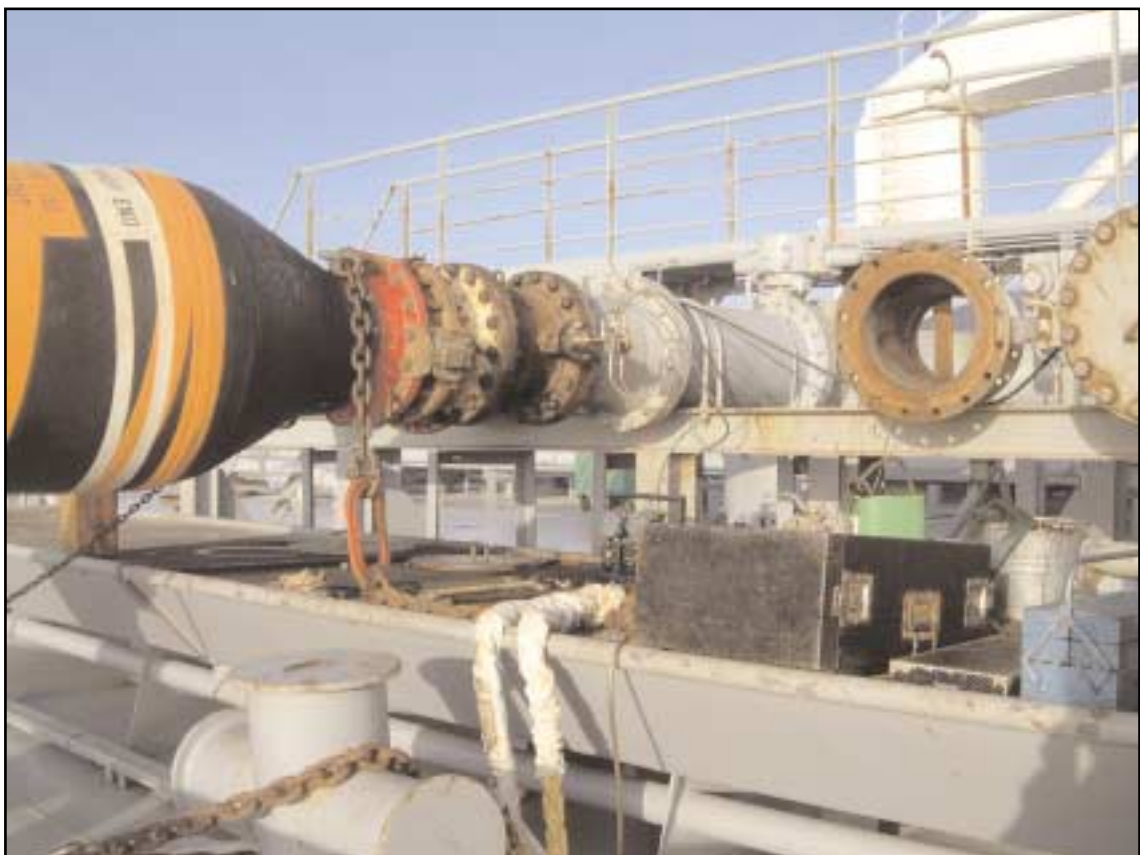
Discharge manifold showing couplings and safety chain
