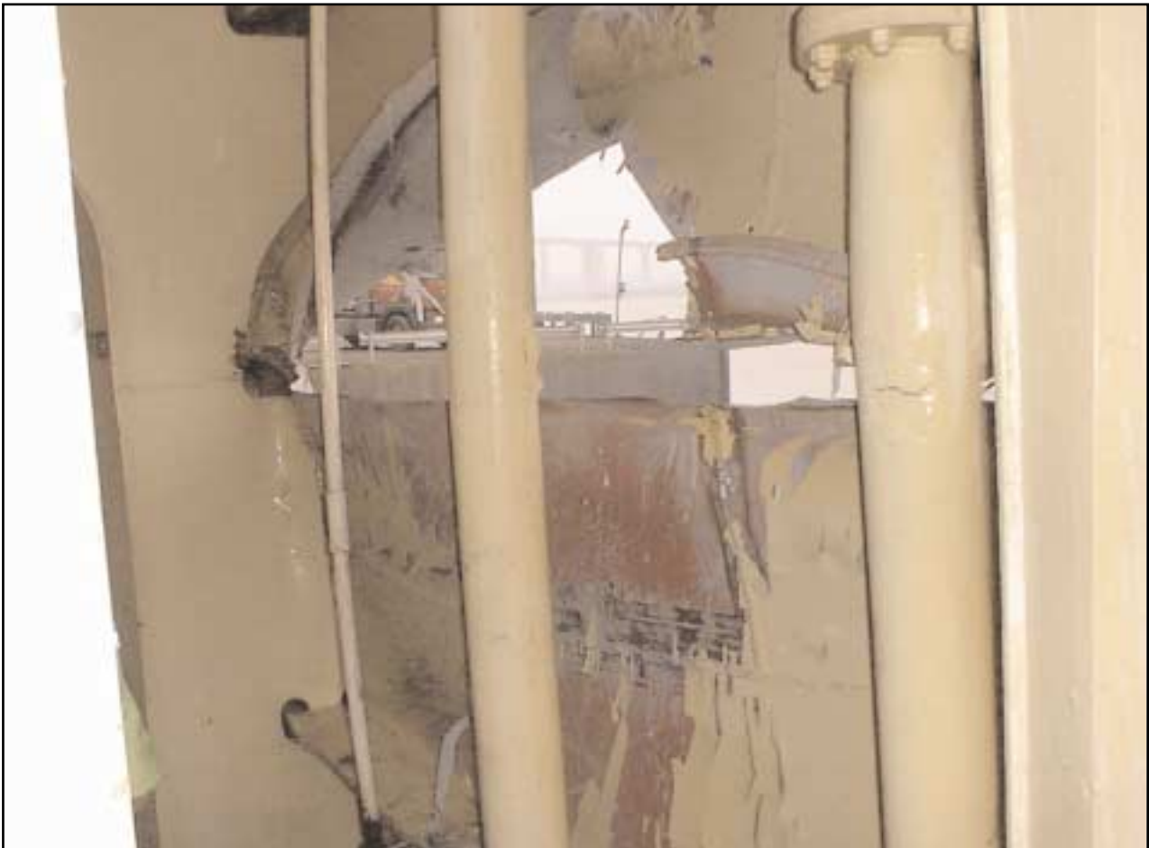
Internal view of damage to Loverval
