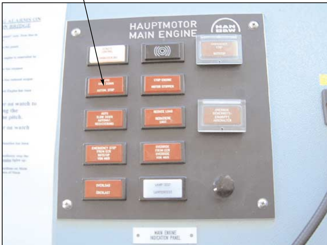
Bridge console engine alarms
