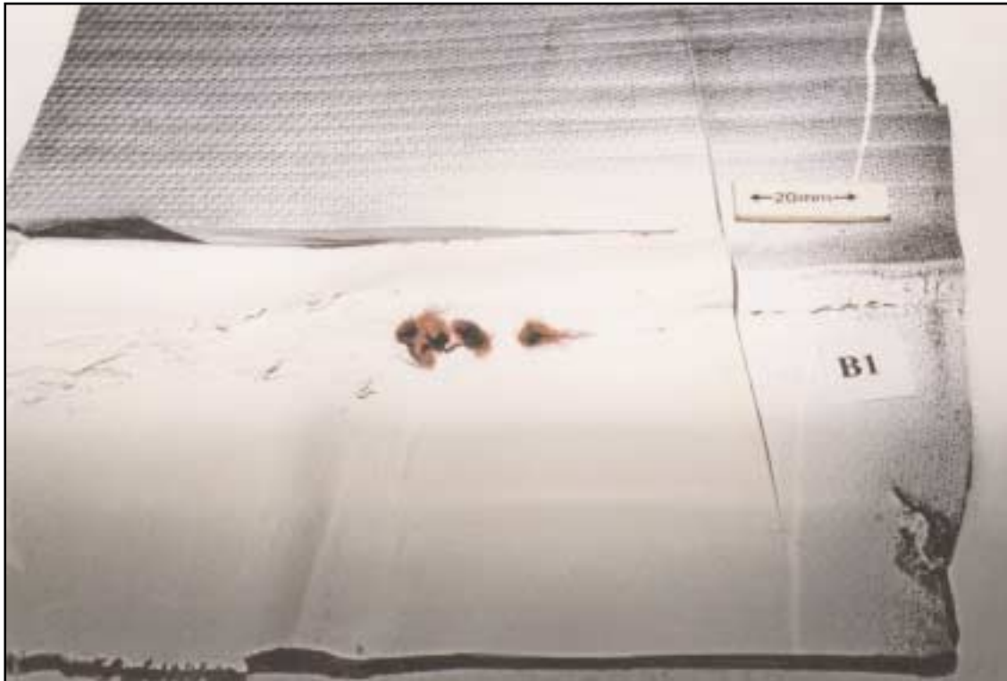
Site of liner perforation identified by dye penetrant test
