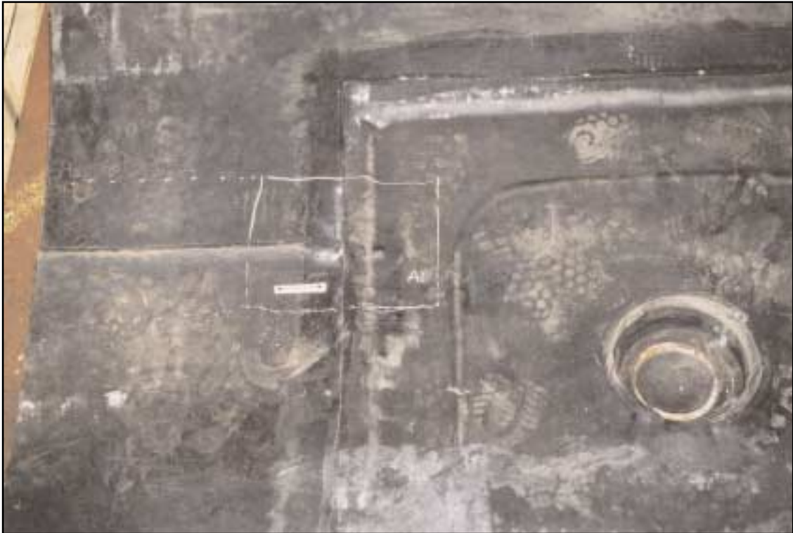
'T' joint in liner
