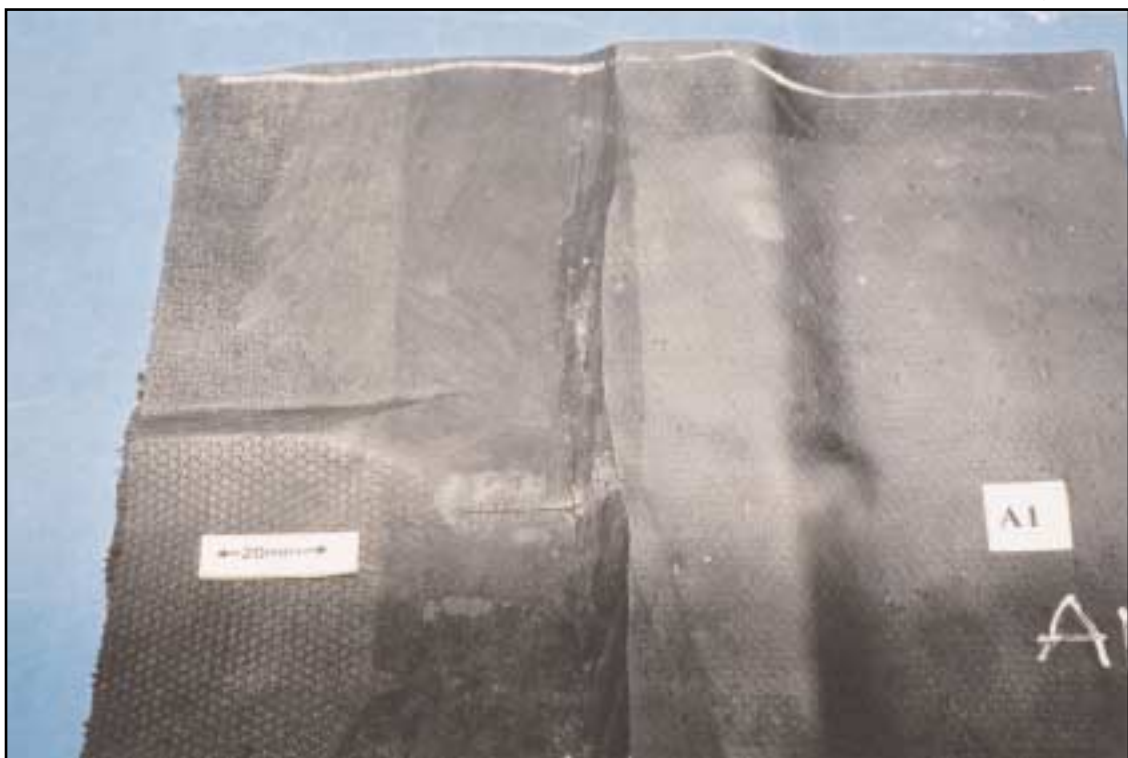
Cut in butyl liner (lower centre of figure)
