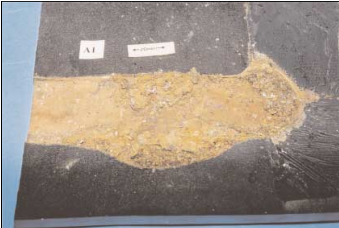
Shell corrosion in region of liner's 'T' joint
