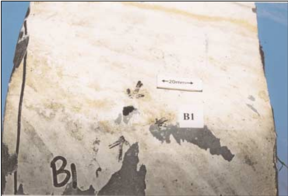
Second leak site - view on outer surface
