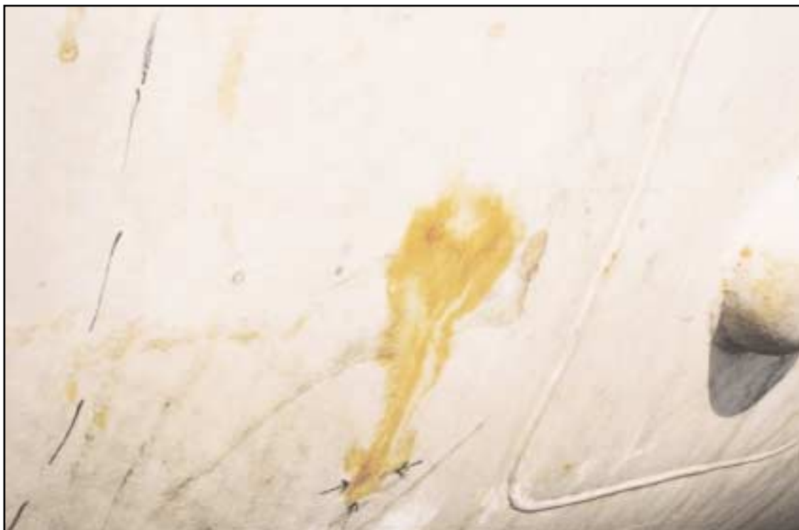
Site of leakage and associated rust staining
