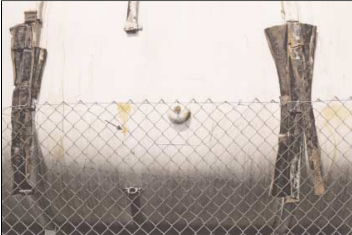
Site of leakage, shown arrowed
