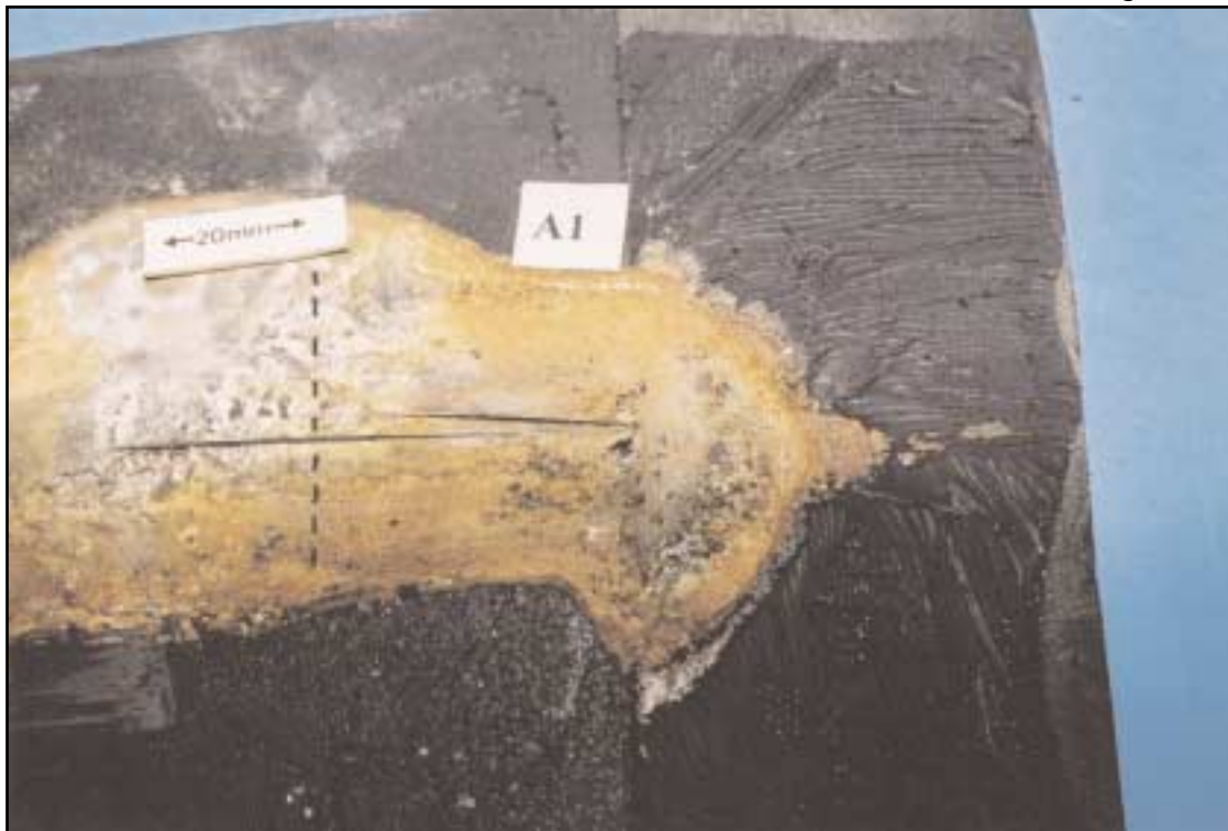
Cuts in underside of butyl liner
