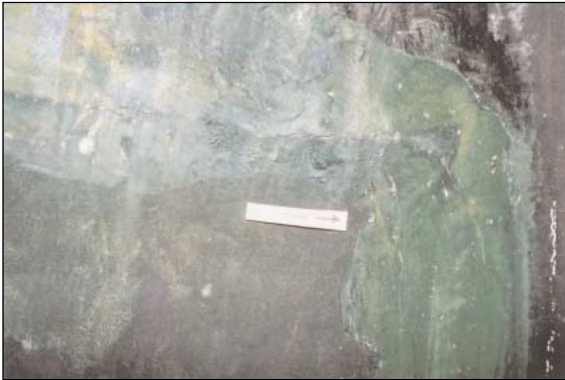
Cracking in resin material used for repairs
