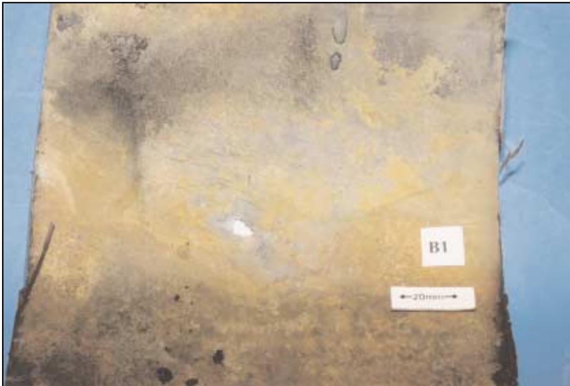
Second leak site - view on inner surface
