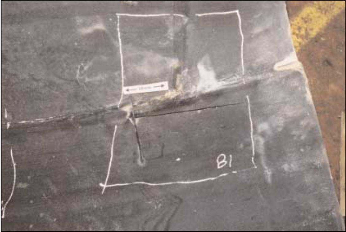
Second leak site
