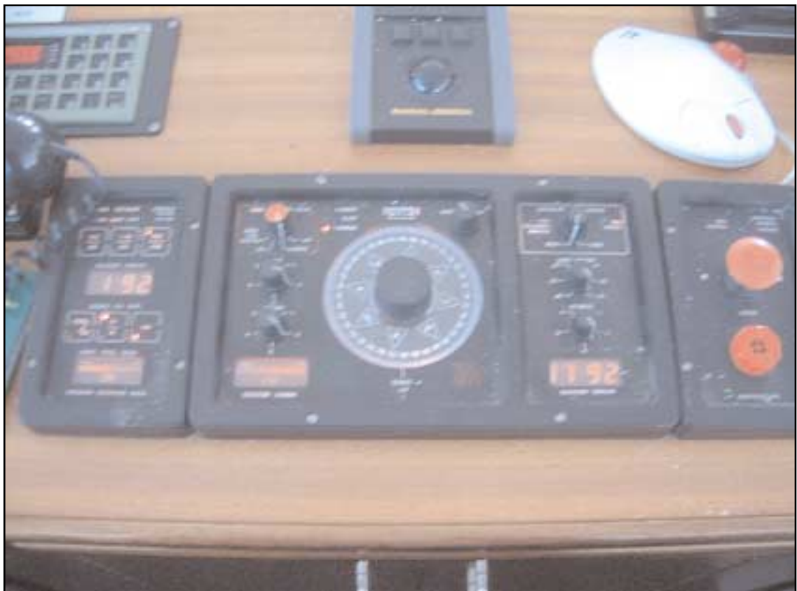
The autopilot (looking aft)
