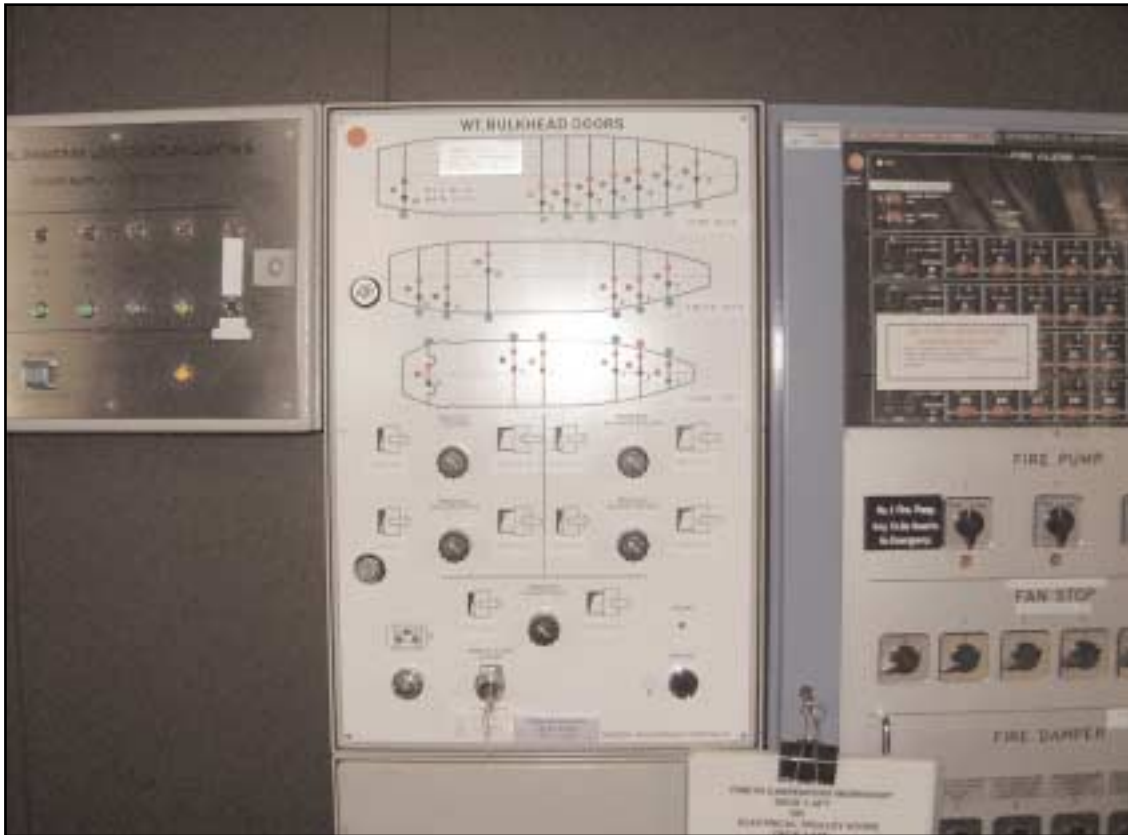
The watertight door mimic board
