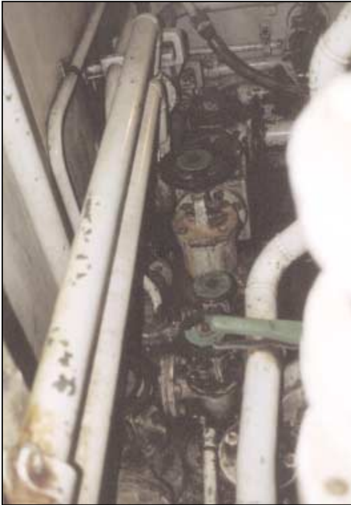
Sea water inlet valves - port side main engine well
