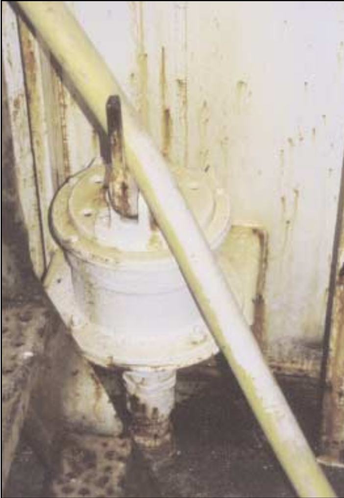
Engine room bilge hand pump on aft working deck
