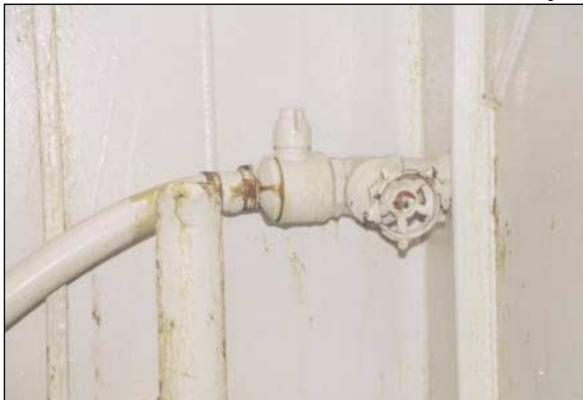
Typical deck wash connection
