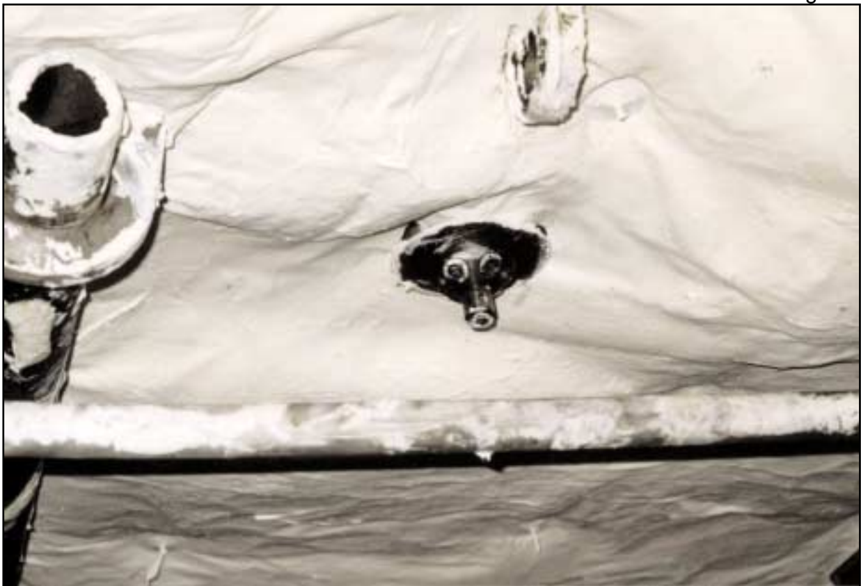
Hi fog head above generator No 3
