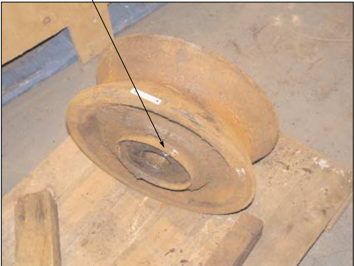
A view of the roller, showing the extent of the outward movement of the steel sleeve from the bearing housing
