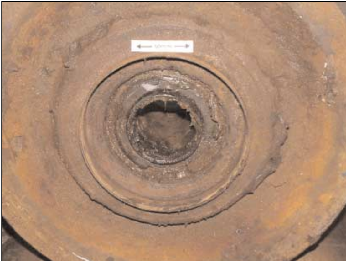
Closer view of inboard side of roller showing fractures to inner and outer ball races
