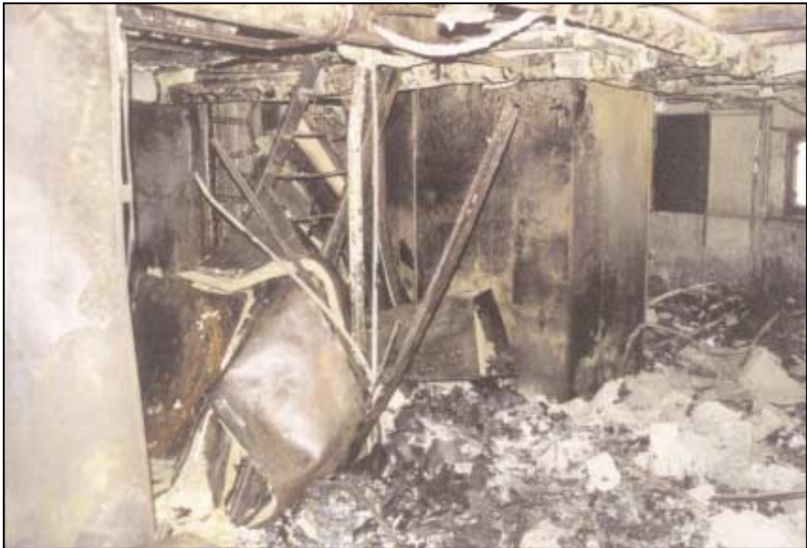
General view of fire damage of deck
