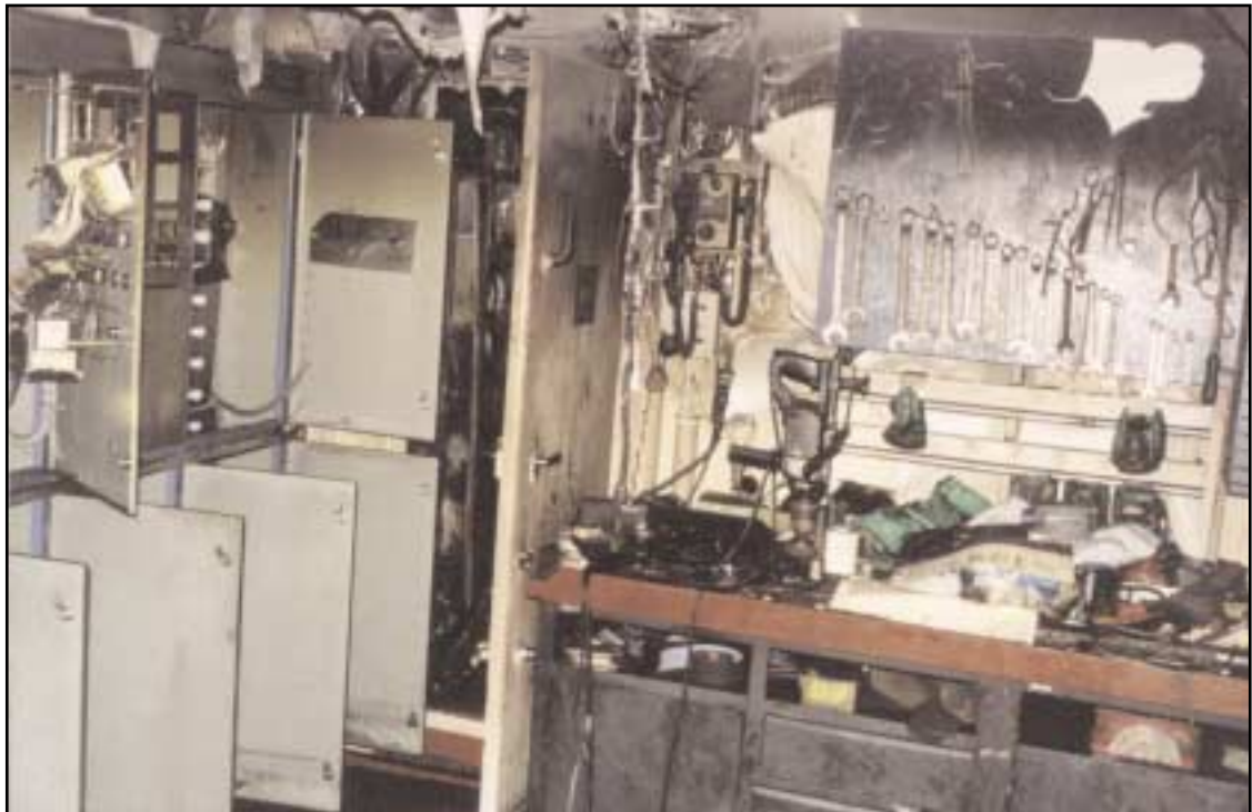
Engine workshop showing damaged deckhead Note: lack of fire damage to items on workbench
