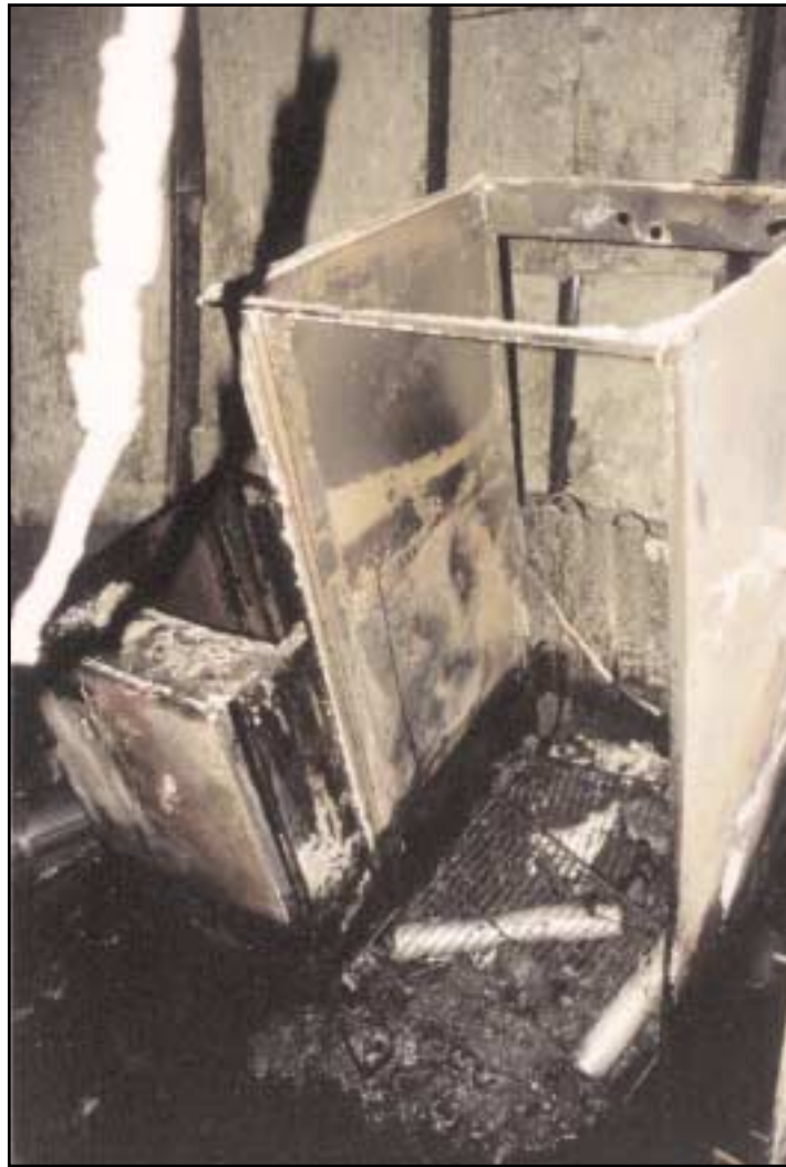
Remains of fire damaged upright freezer
