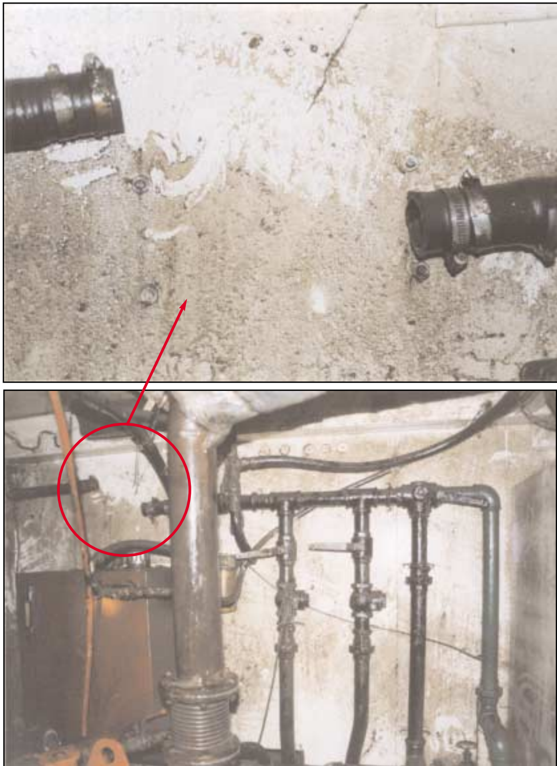
View of aft engine room bulkhead showing location of missing manual bilge pump
