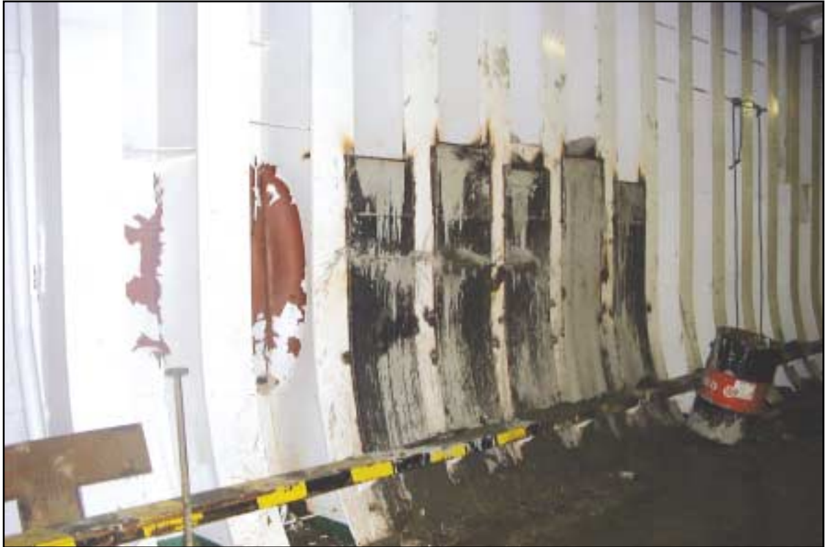
Temporary repair made to damage
