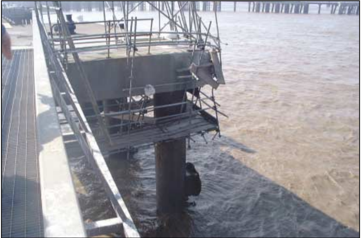
Fender 24 (note damage to scaffolding)
