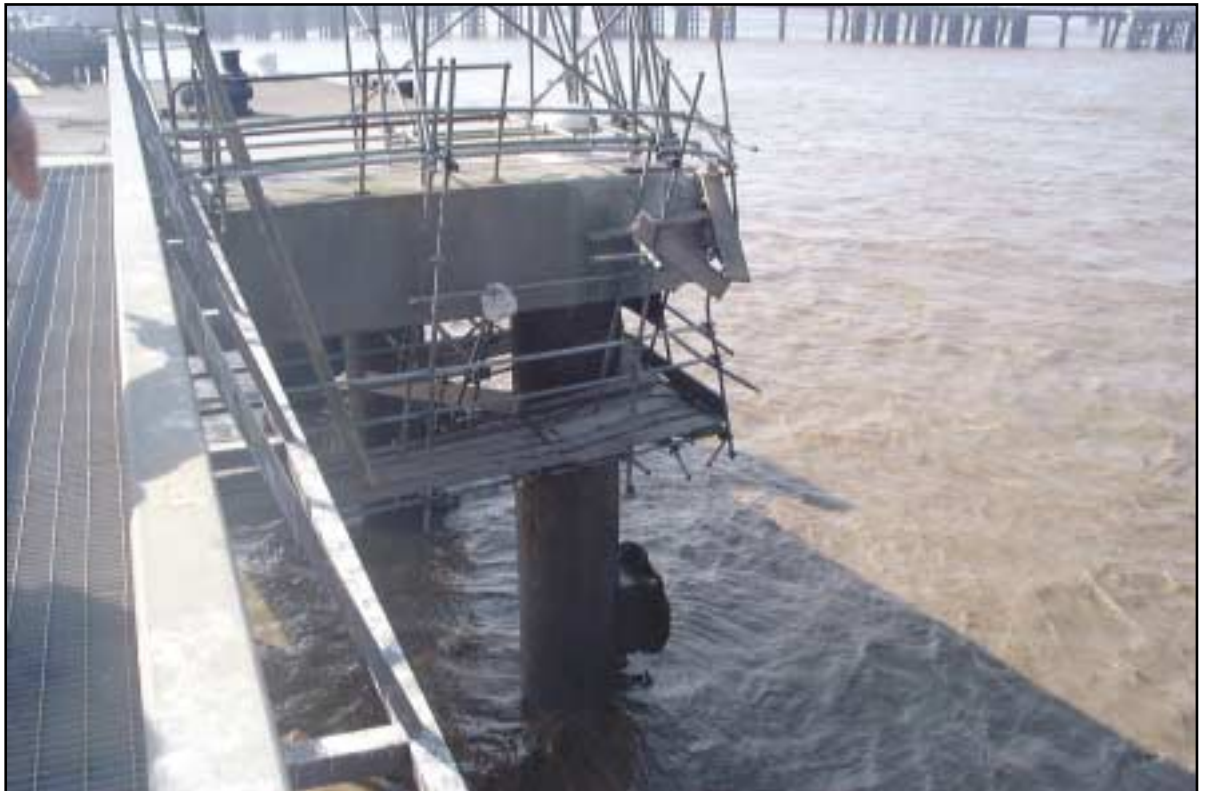
Fender 24 (note damage to scaffolding)
