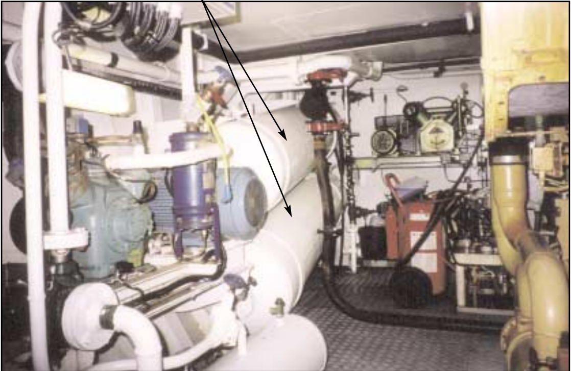
Forward / port corner of engine room
