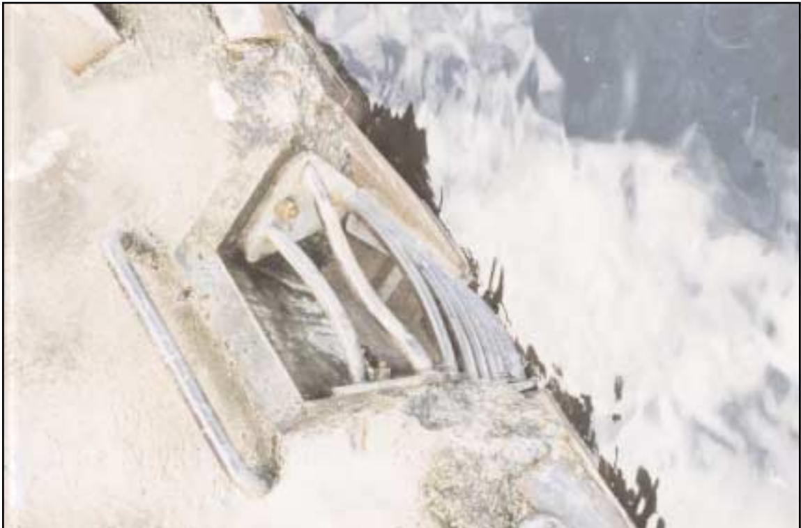
Market quay ladder concerned
