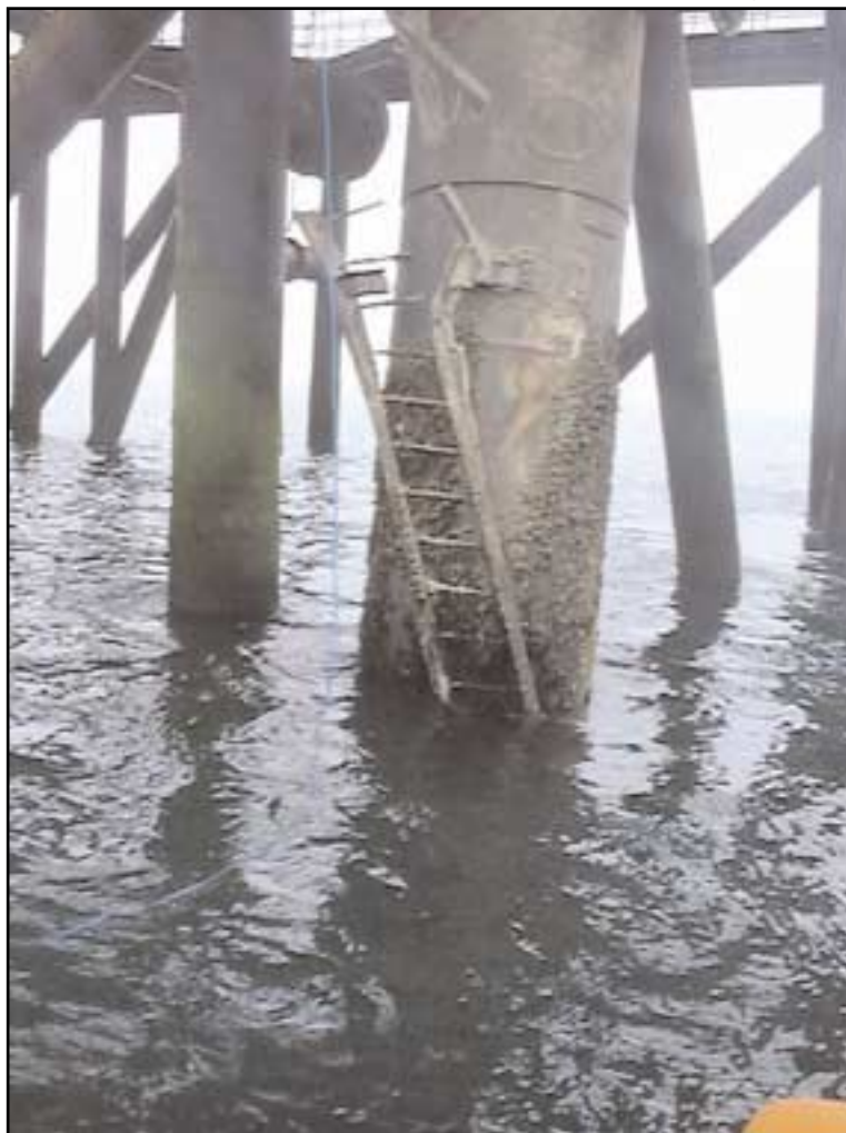
Close view of damage to BD jacket
