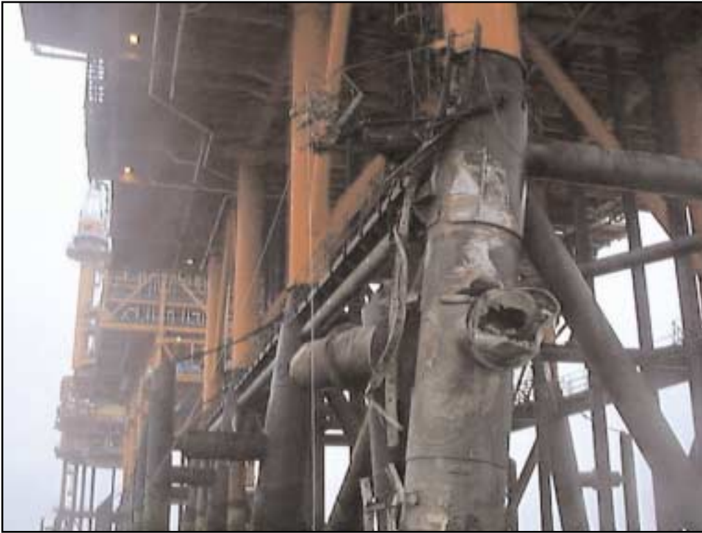
General view of damage to BD jacket
