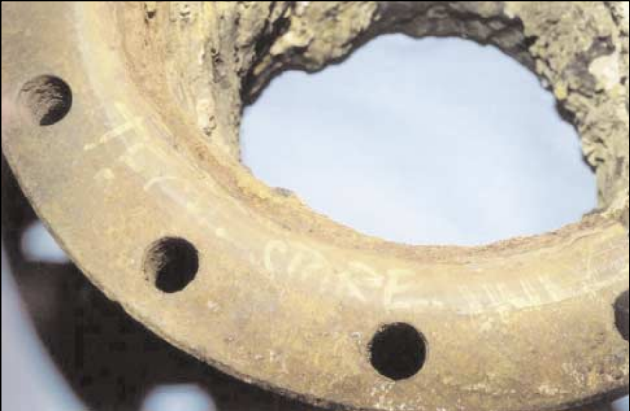
Corrosion damaged pipe end, and absence of any remnants of the inner flange to pipe sealing fillet weld. Heavy marine growth and corrosion products at top of picture
