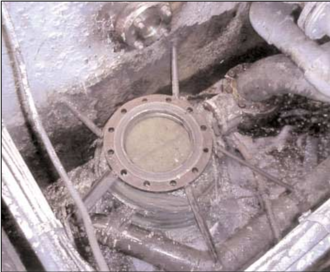
Reinforcing stays between valve flange and surrounding structure (inboard piping and strainer removed)
