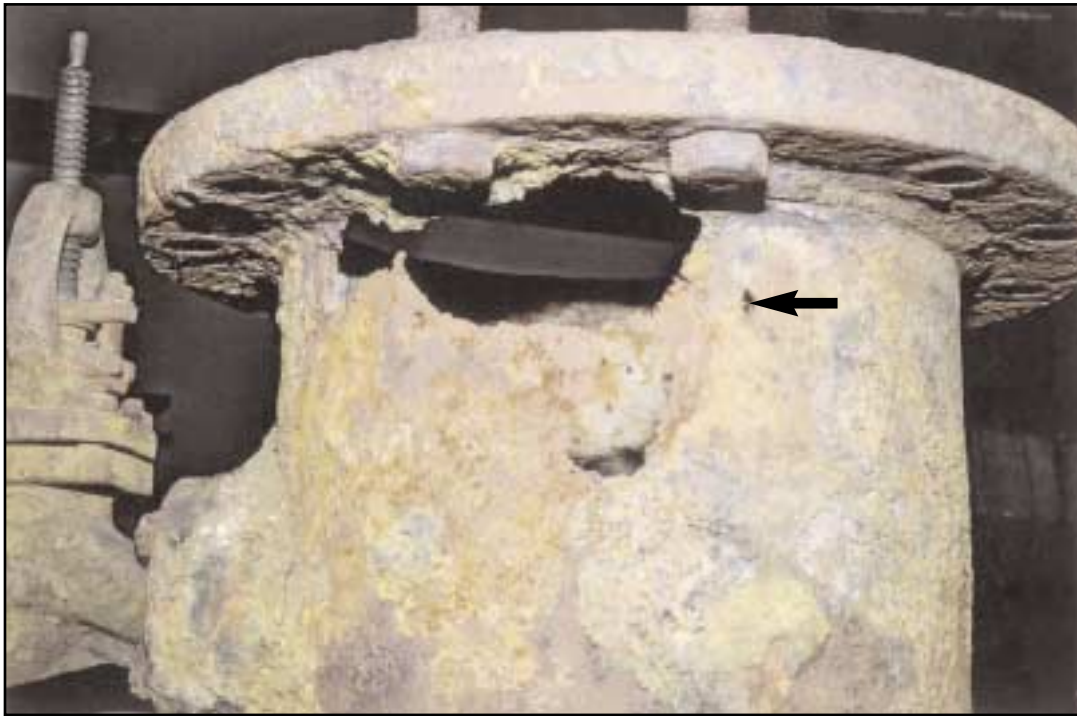
Detail of principal leak site showing corrosion of flange underside and local loss of the outer flange to pipe fillet weld. The figure also shows a close proximity secondary pipe wall perforation site (arrowed)
