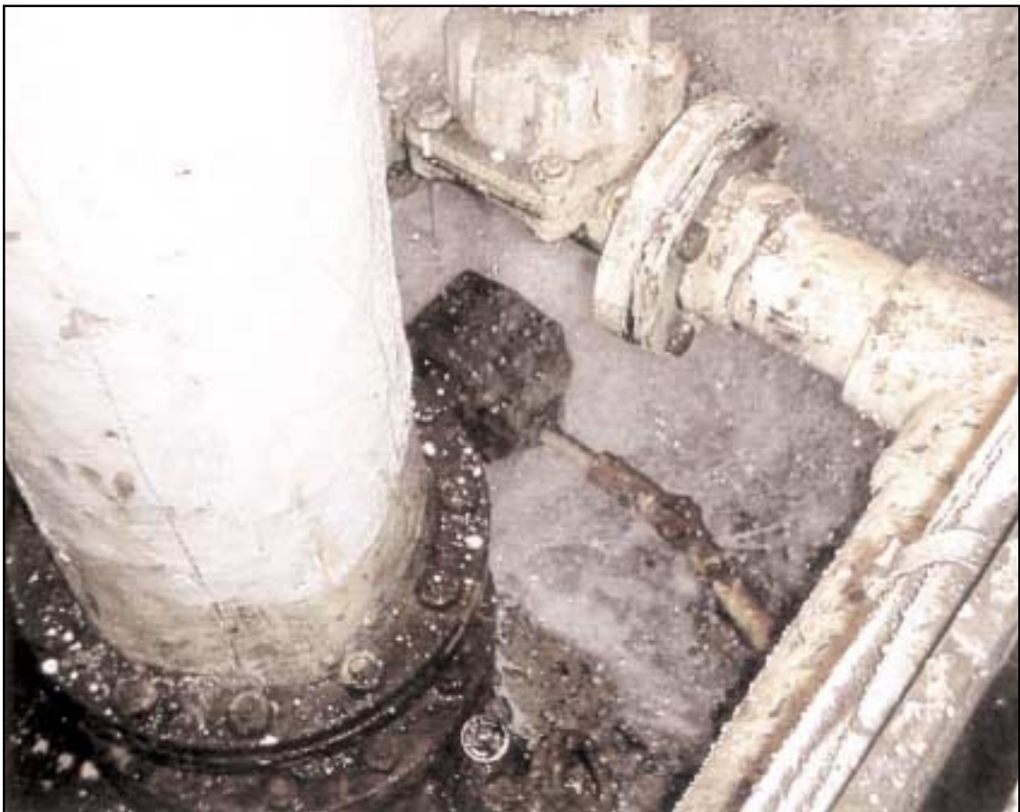
Leak from 250mm sea inlet
